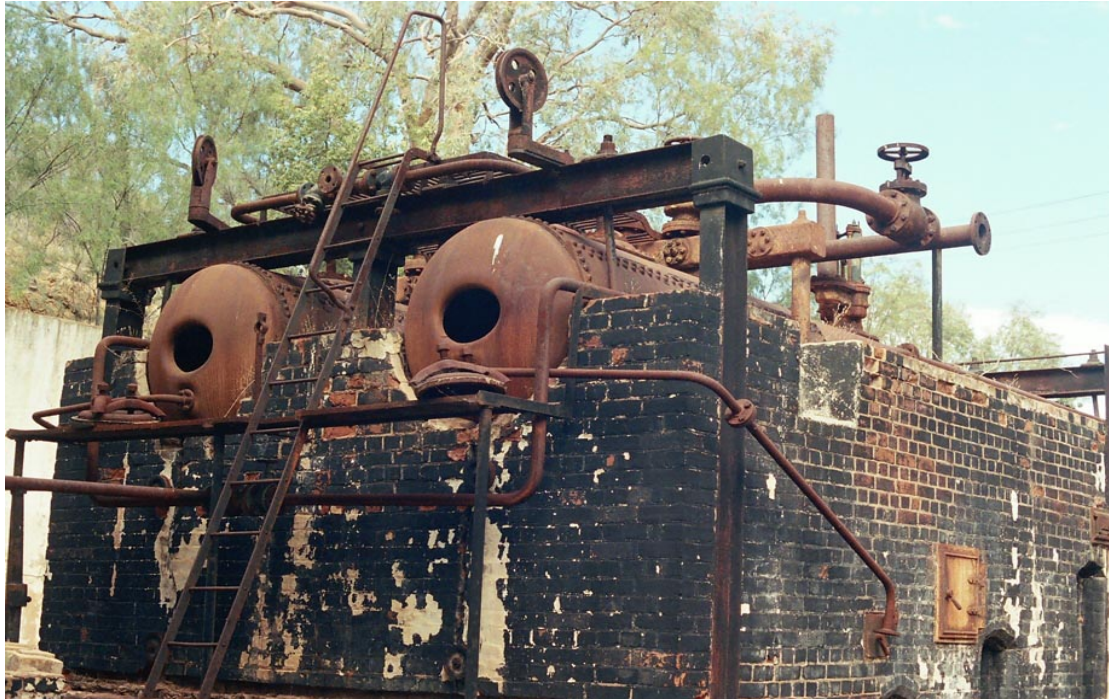
Plate 5. Umberumberka Pumping Station. Two Babcock and Wilcox water tube boilers which supplied steam to the Hathorn Davey pumping engines.
