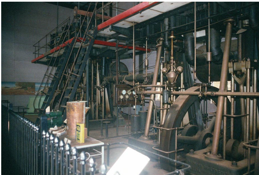
Plate 2. Umberumberka Pumping Station. The two Hathorn Davey triple expansion vertical inverted steam pumping engines.
