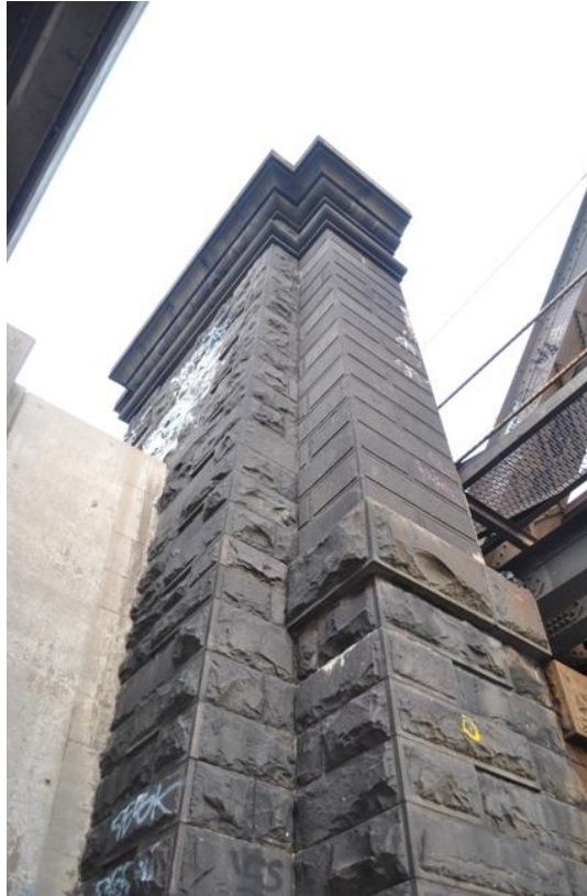
The original bluestone abutment and tower of the Saltwater River Bridge. The construction is of very high quality.
