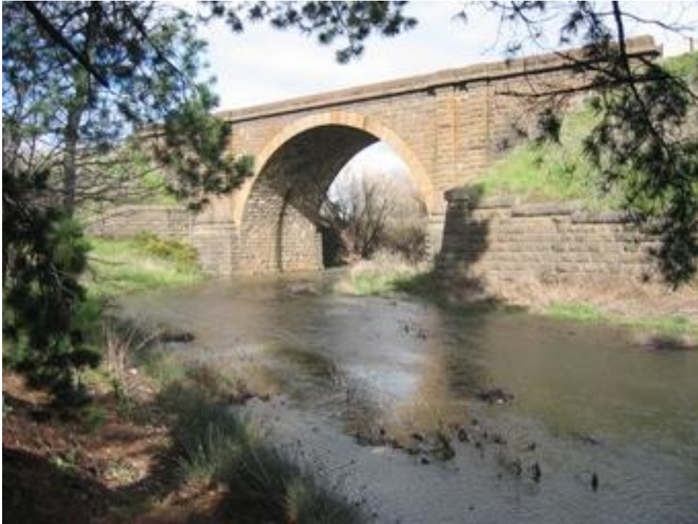
Riddells Creek Bridge. Typical of the many stone bridges on the line.
