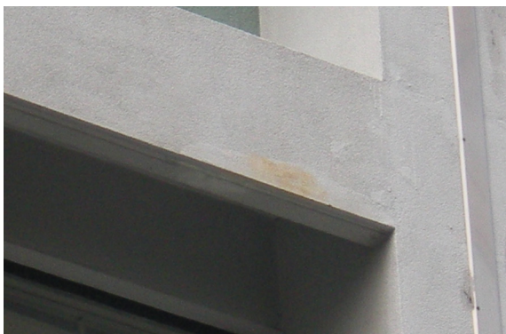
Staining on the West Wing
