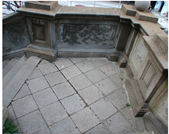
Concrete repairs and gaps in the paving of the Battery Path steps
