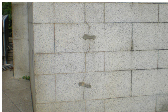
Cracks in the granite walling
