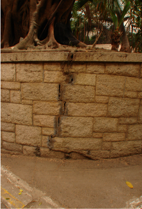
A large crack in a retaining wall for a flower bed
