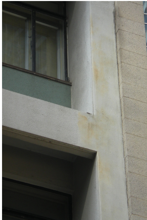
Staining on the West Wing
