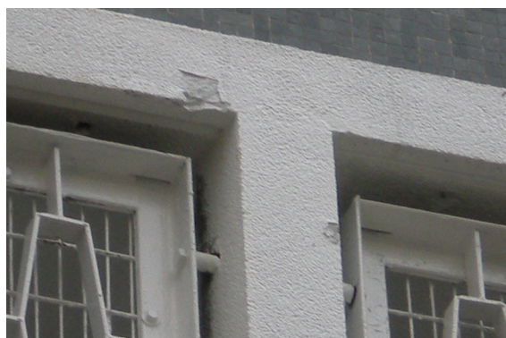
Spalling to the concrete of the Central Wing
