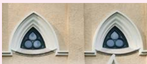
為適應香港亞熱帶氣候而設計的可開啟的三葉草形窗 Openable trefoil windows adapted to the sub-tropical climate in Hong Kong
