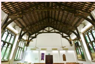
由兩組托臂梁支撐的中式金字瓦頂 A Chinese tiled pitched roof supported by double hammer-beam timber roof trusses
