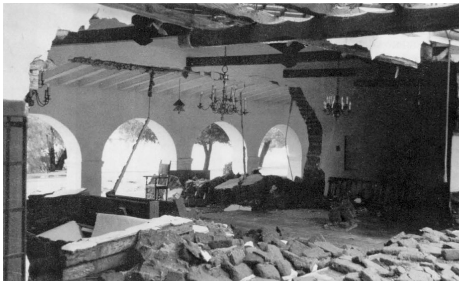
The chapel of the Camp Pendleton Ranch House, scene of many Marines' weddings and other rites of passage since the middle of this century, was devastated when the levy behind the Ranch House burst, and east and west facing walls of the chapel collapsed.
