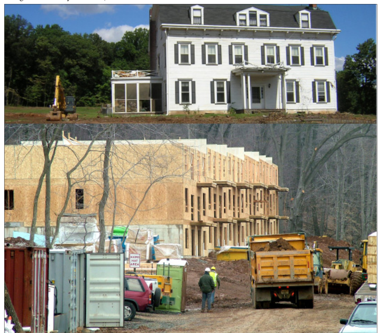
NEW CONSTRUCTION...Construction of condominiums by K. Hovnanian is underway in Scotch Plains between Route 22 and Diamond Hill Road. Inset is a photo of the house that previously stood on the property. Residents had objected to the construction, citing drainage problems in the area.
