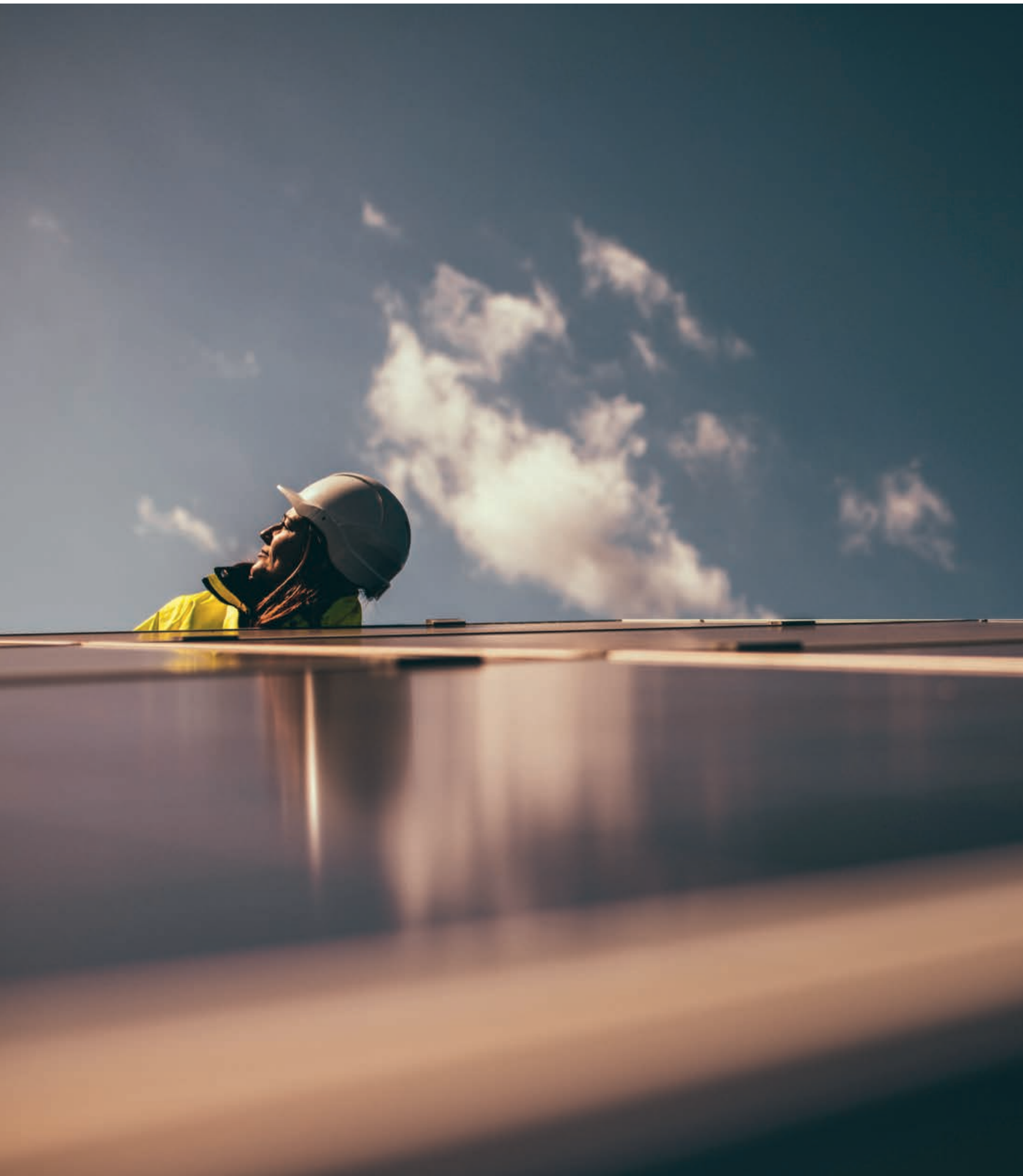
Photo by Arlindo Camacho, Photovoltaic installation - Portugal, 2018
