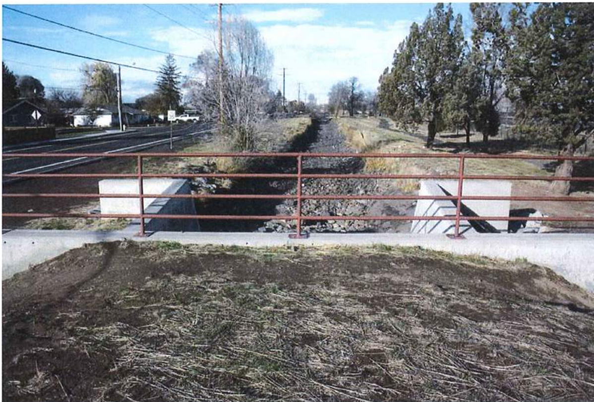
Photo 7 of 49: Pilot Butte Canal: Downtown Redmond Segment Historic District, looking north from top of outlet structure
