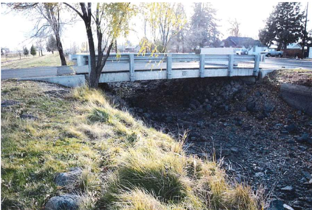
Photo 10 of 49: Pilot Butte Canal: Downtown Redmond Segment Historic District, NW Fir Avenue bridge, looking southwest
