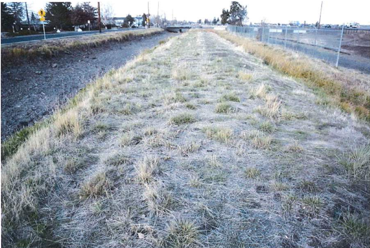
Photo 20 of 49: Pilot Butte Canal: Downtown Redmond Segment Historic District, looking north across east embankment towards NW Hemlock Avenue
