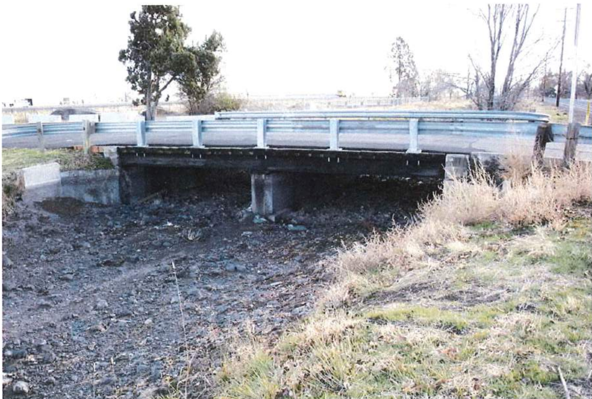
Photo 24 of 49: Pilot Butte Canal: Downtown Redmond Segment Historic District, NW Hemlock Avenue bridge, looking northwest
