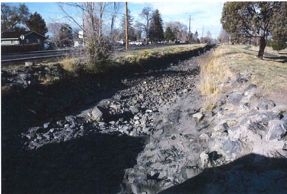
Photo 8 of 49: Pilot Butte Canal: Downtown Redmond Segment Historic District, looking northwest from east side of outlet structure
