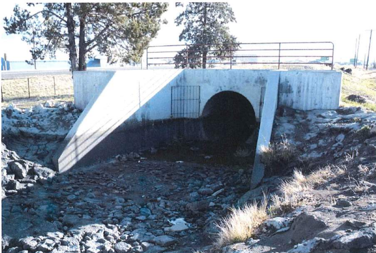
Photo 6 of 49: Pilot Butte Canal: Downtown Redmond Segment Historic District, outlet structure, looking southeast
