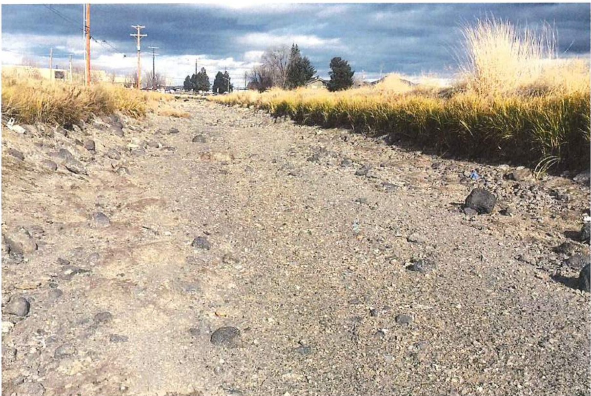
Photo 28 of 49: Pilot Butte Canal: Downtown Redmond Segment Historic District, looking north to NW Kingwood Avenue bridge
