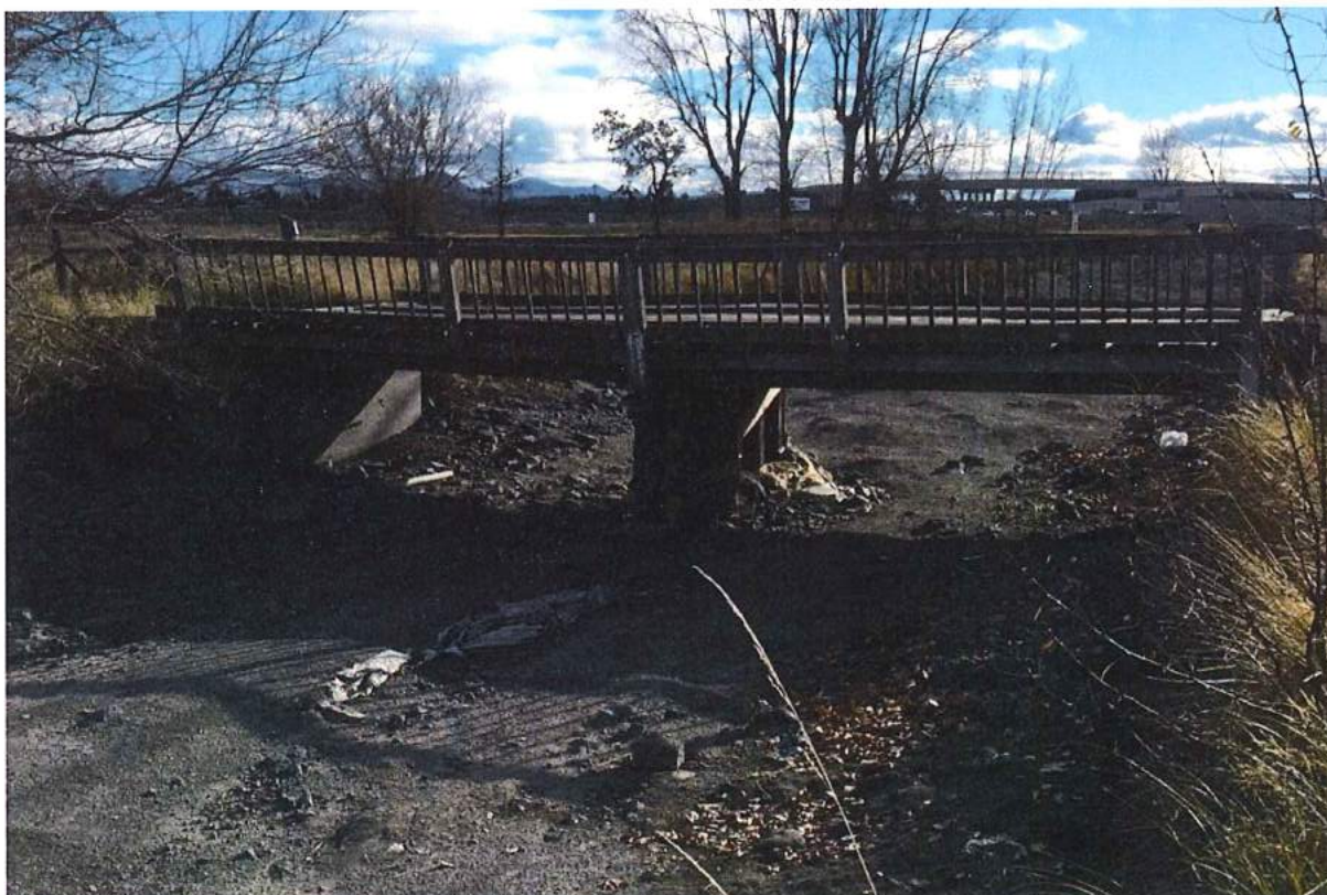
Photo 46 of 49: Pilot Butte Canal: Downtown Redmond Segment Historic District, 2036 NW Canal Boulevard bridge, looking southeast
