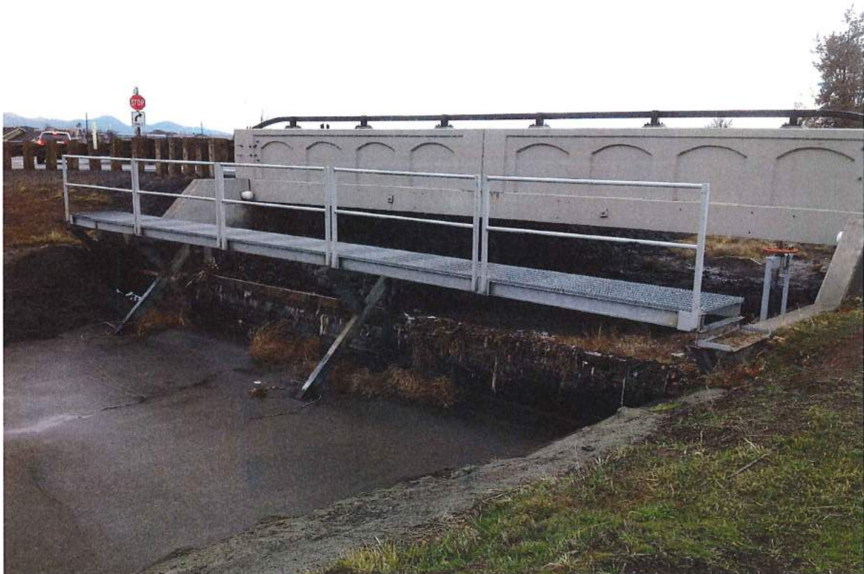
Photo 36 of 49: Pilot Butte Canal: Downtown Redmond Segment Historic District, Check Structure, Lateral D Headgate, and NW Larch Avenue bridge, looking southeast
