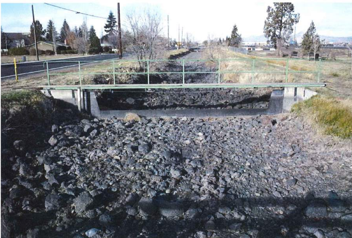
Photo 16 of 49: Pilot Butte Canal: Downtown Redmond Segment Historic District, weir, looking north from NW Greenwood Avenue bridge
