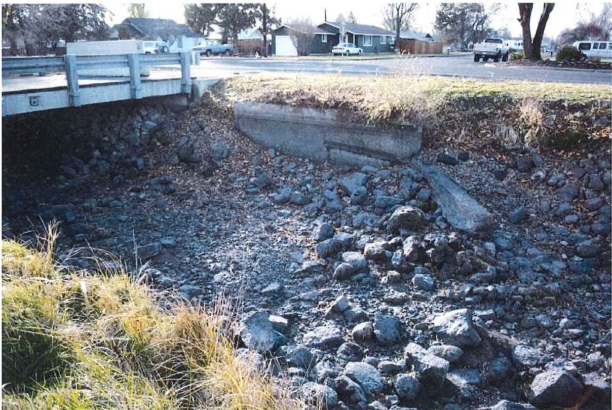
Photo 12 of 49: Pilot Butte Canal: Downtown Redmond Segment Historic District, Lateral D-2 headgate, looking southwest
