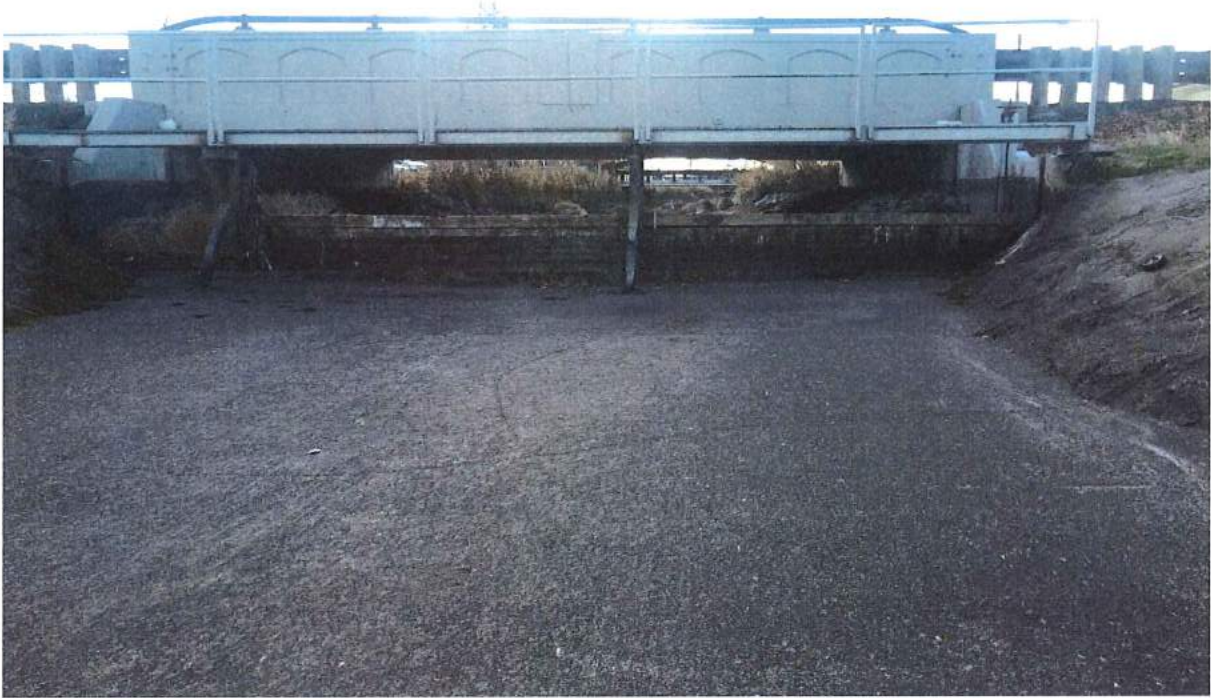
Photo 39 of 49: Pilot Butte Canal: Downtown Redmond Segment Historic District, Check Structure and NW Larch Avenue bridge, looking southwest
