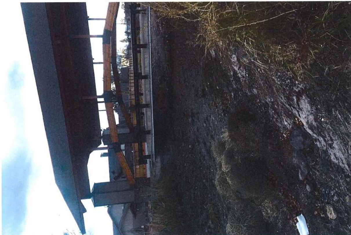
Photo 34 of 49: Pilot Butte Canal: Downtown Redmond Segment Historic District, Medical Center bridge, looking south
