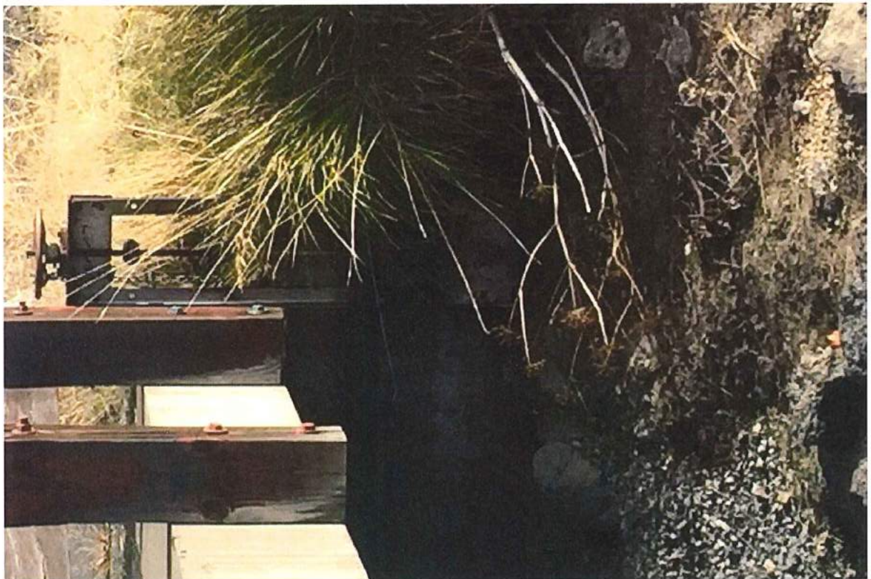
Photo 30 of 49: Pilot Butte Canal: Downtown Redmond Segment Historic District, headgate next to NW Kingwood Avenue bridge, looking east
