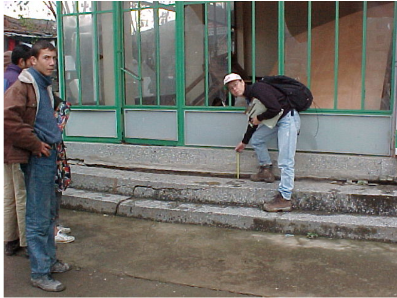
Figure 11. Localized ground settlement of 1 cm adjacent to building (N40.8389, E31.1548)
