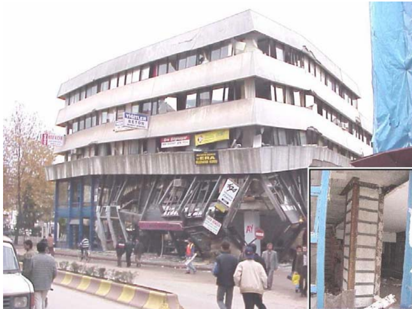
Figure 15. Building in Duzce that had been retrofitted after the 1999 Kocaeli earthquake (N40.5034, E31.0952)
