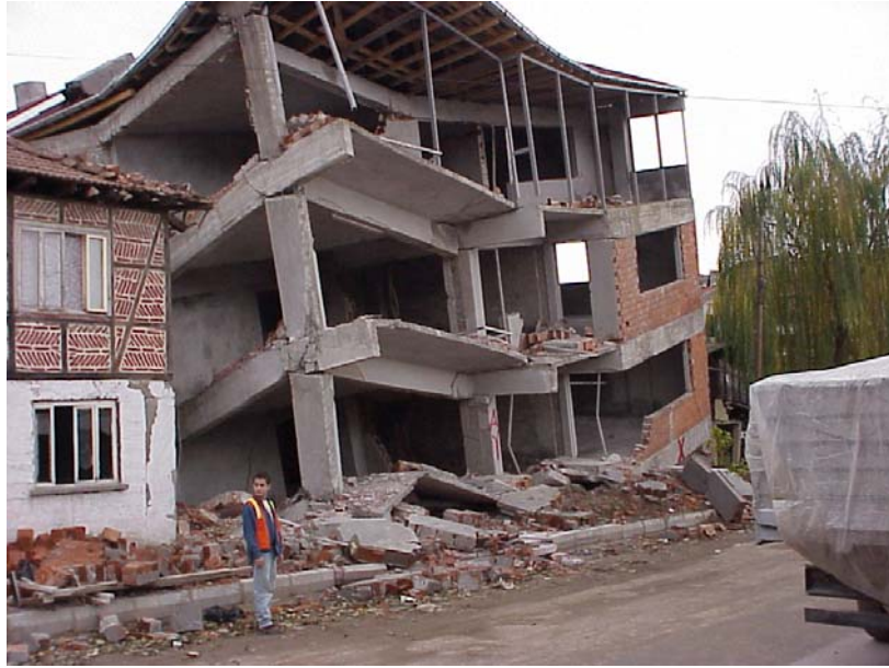
Figure 17. Example of poorly reinforced structure with no bonding between structural members in Kaynasli (N40.4631, E31.1923)
