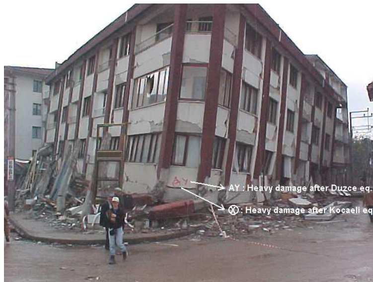
Figure 12. Collapsed building in Duzce that had already been damaged during the Kocaeli event (N40.83678, E31.1582)
