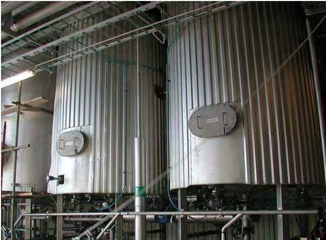
Figure 10. Pasteurisation tanks at the Uppsala biogas plant.
