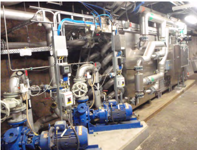
Figure 4. Two new tube heat exchangers installed in parallel below one of the anaerobic digesters, photo by Ulf Jansson, BYAK AB.
