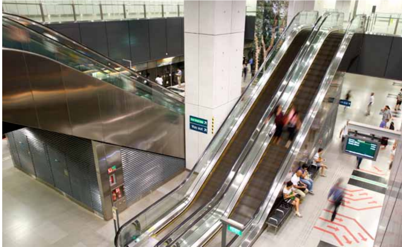
Ensuring that escalators at our MRT stations are safe and reliable is a priority.
