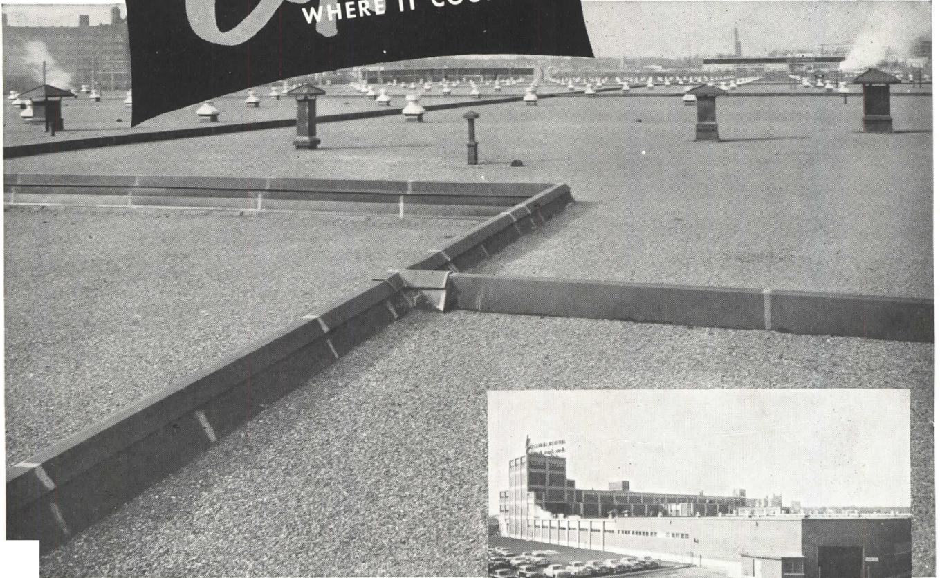
ACRES AND ACRES of roof with 4,000 ft. of 4 ft. girth, 20-oz. Revere Copper expansion joints guarding against an invasion by weather. Non-rusting, enduring Revere Copper was also used for the fascia, ventilators and for flashing around the rising walls.
