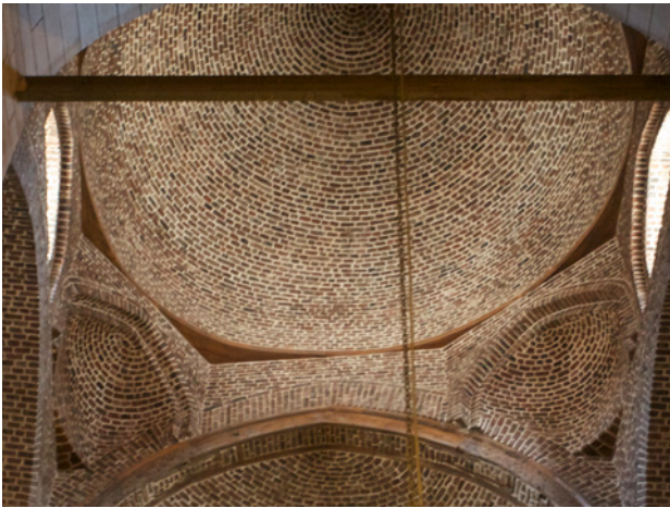
Fig. 2. Dome of the Church of Saint Mercurius (Dayr Abu Sayfayn), Cairo. (Photo: Jennifer Pruitt)
