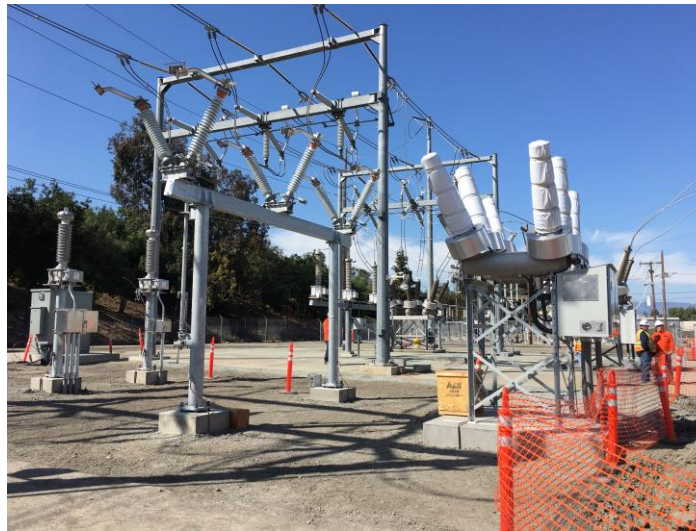
New 115kV Breaker on Pad
