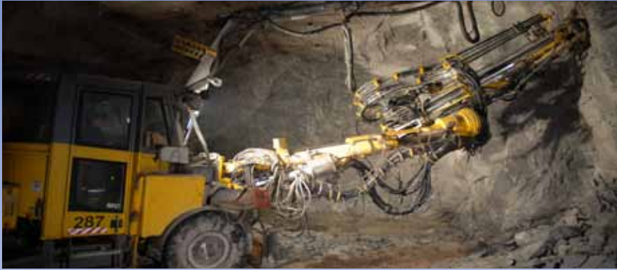
In one of Diavik Diamond Mine's underground tunnels, a bolt operator attaches a screen. Photo Courtesy of Diavik Diamond Mines Inc.
