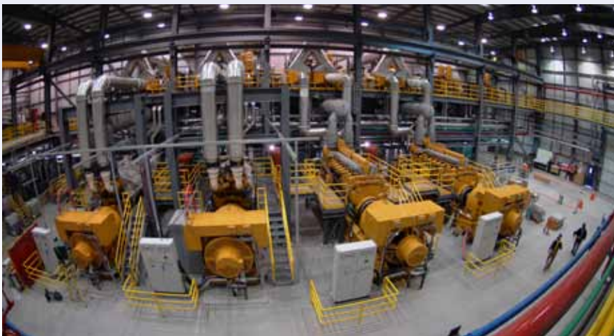
As part of the underground mine construction, Diavik Diamond Mine needed to construct new surface works including a second power house. Photo courtesy of Diavik Diamond Mines Inc.
