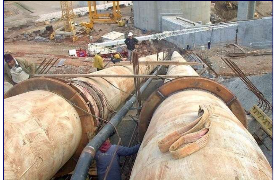
Station de transfert de Beni Haroun
