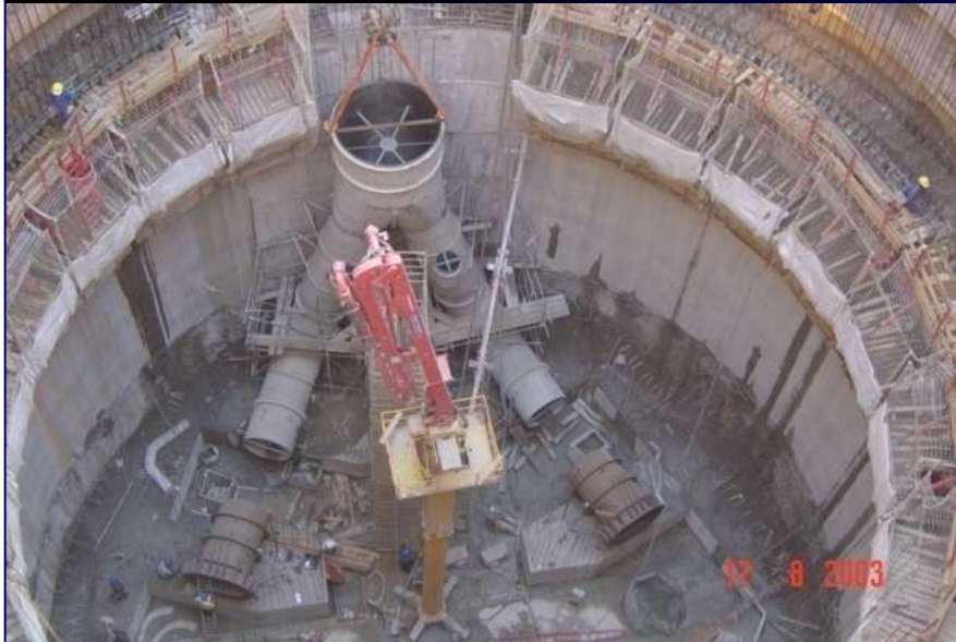
Station de transfert de Beni Haroun
