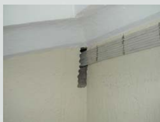
Route of wiring was carefully considered with mock-ups to induce minimum effect.
