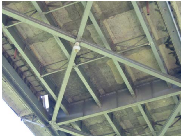
Photo—4.35 Remnants of repairs to concrete slabs
