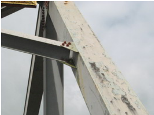
Photo-4.55 Rust of the truss
