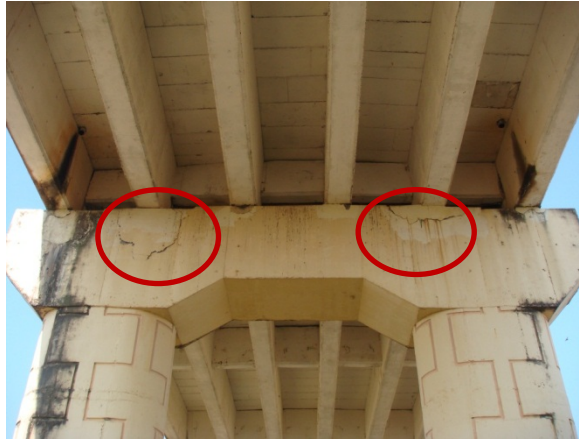
Photo—4.81 Concrete peeling of the cross beam of the H5 pier
