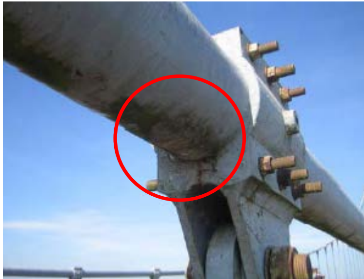
Photo-4.73 Water trace at main cable lapping
