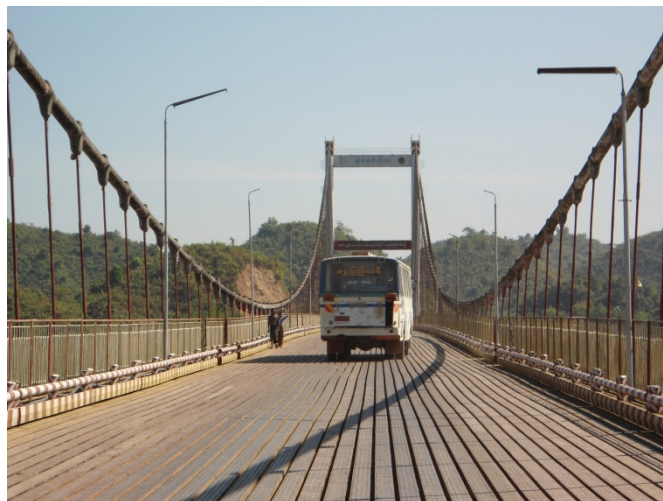
Deformation of steel deck
