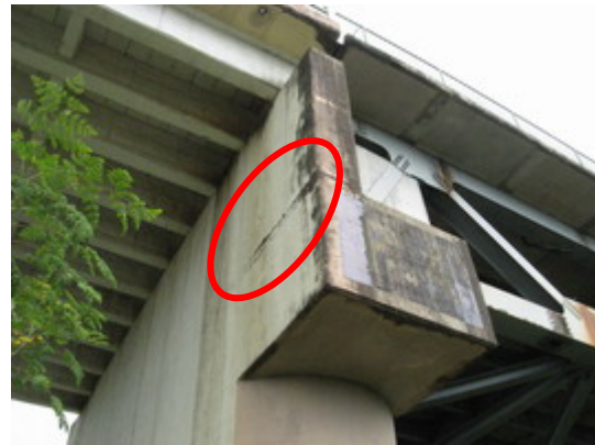
Photo-4.46 Concrete cracks
