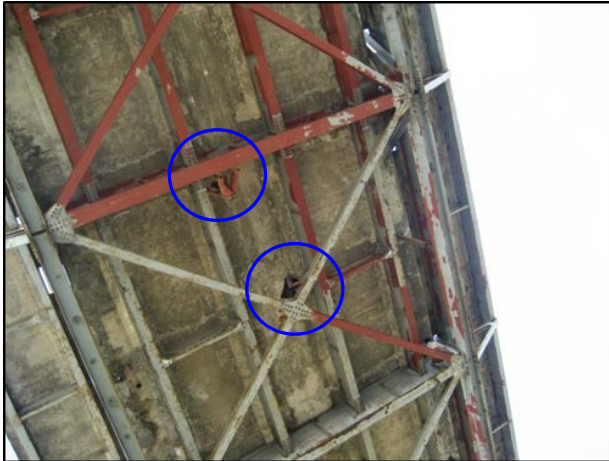
Photo-4.64 Repairing work (within the circle are workers using only a safety rope)
