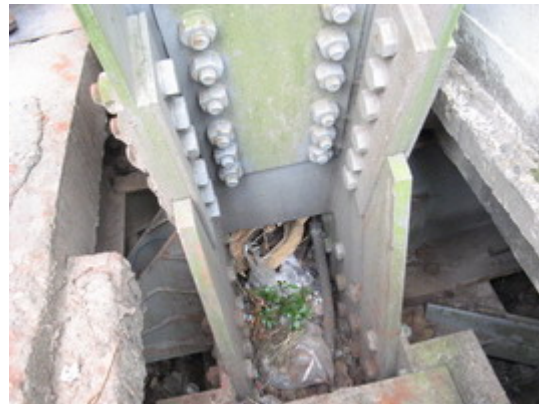
Photo-4.16 Dust at panel point
