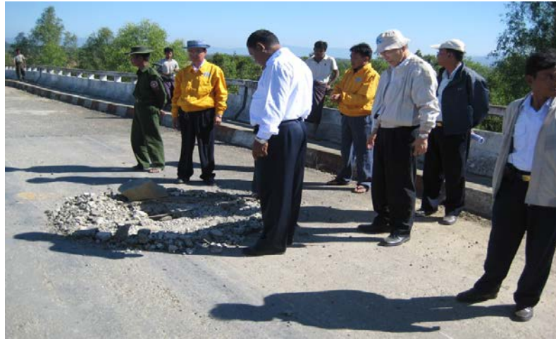
Photo—4.68 Depression in a road surface due to damaged slabs
