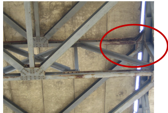
Photo-4.83 Corrosion of the top truss chord
