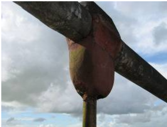
Photo-4.21 Corrosion proofing by cement mortar?
