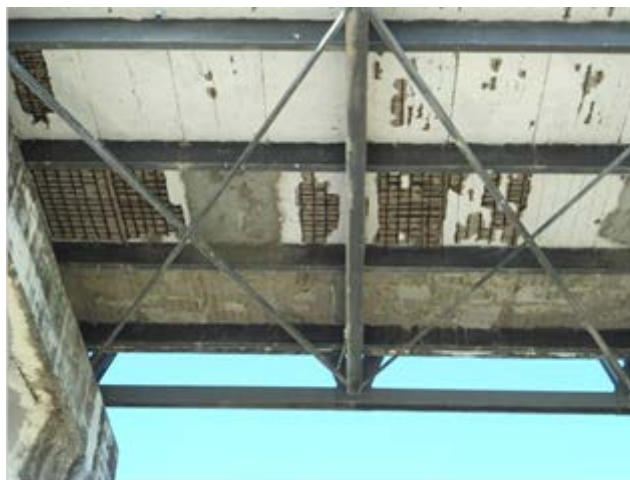
Photo—4.76 Damaged precast concrete slabs
