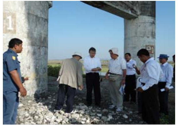
Photo-4.61 Fragments of peeled off concrete around a pier
