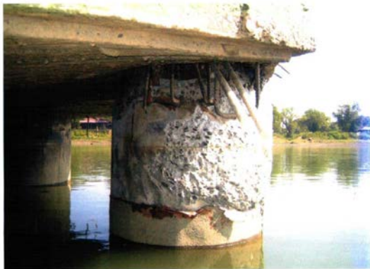
Photo-3.11 Section of poor execution at the pile top
