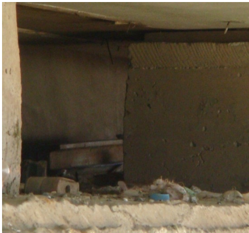
Photo-4.49 Fractured member of expansion joint dropped on the top of the pier
