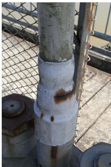
Photo—4.74 Breaking and peeling of the hanger's FRP covering
