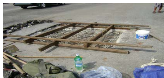
Slab damage due to Heavy truck in Bandoola bridge
