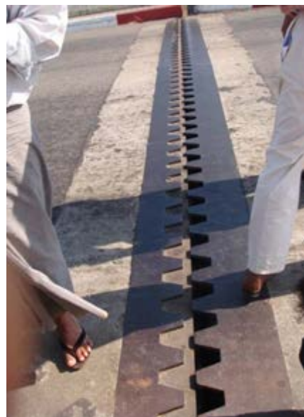
Photo-4.80 Gap of expansion joint 5
