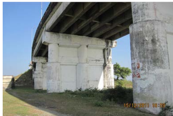
Photo—4.63 Strengthening of the piers of the Min Chaung Bridge using concrete lining
