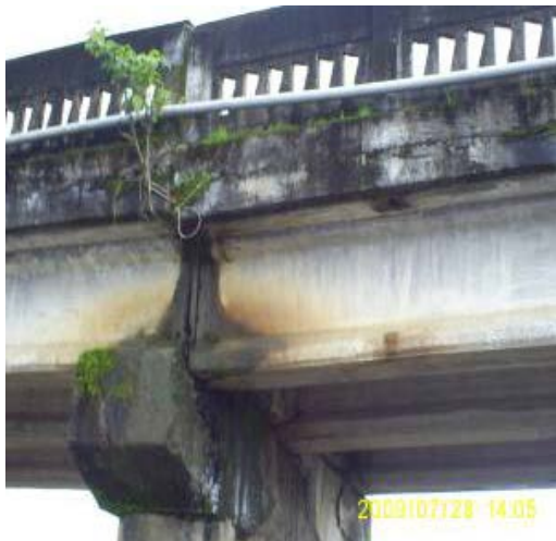
Photo-4.4 Concrete girder nearly falling from substructure
