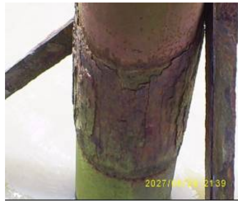
Photo-3.10 Deterioration of pipe
