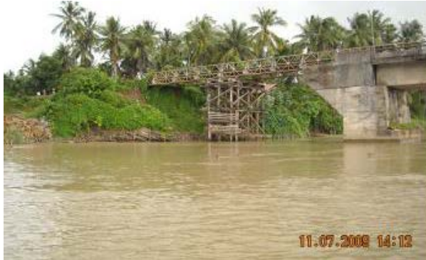
Photo-3.3 Passage of traffic was secured by using a temporary bridge when the rear face of an abutment was scoured during flooding
