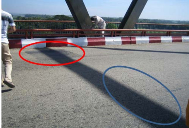
Photo—4.34 Damaged asphalt pavement
