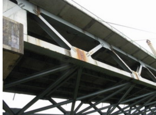
Photo-4.42 Rust due to drain water from the road surface
