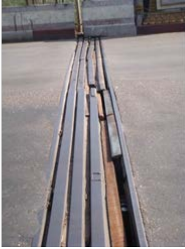
Photo-4.47 Damage to an expansion joint
