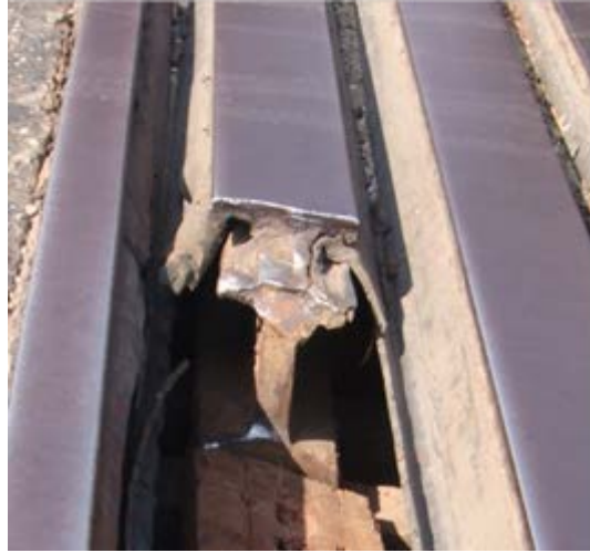
Photo-4.48 Fractured member of expansion joint
