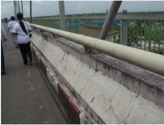
Photo-4.45 Cracks in the bridge railing
