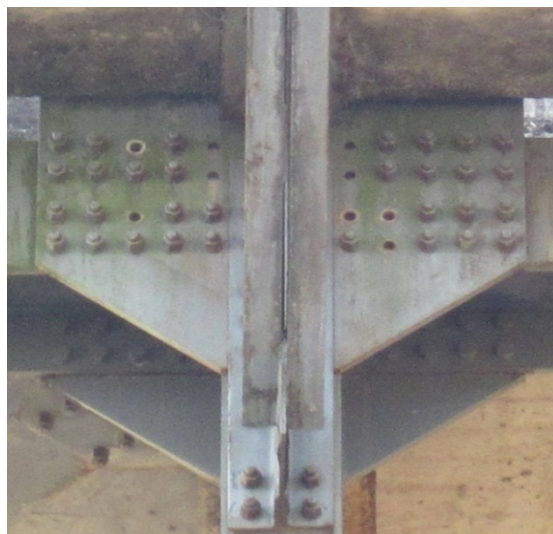
Photo-4.72 Deficit of bolt at truss splice plate
