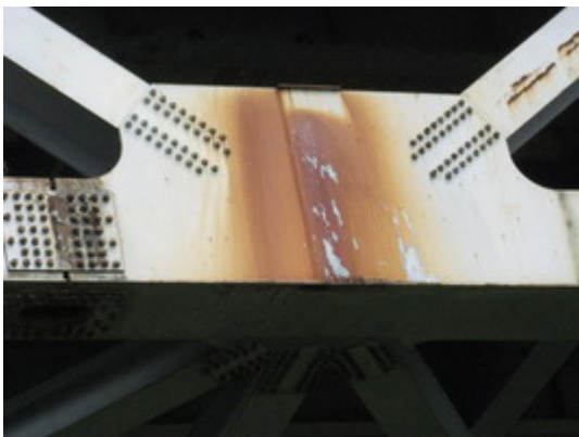
Photo-4.43 Rust due to drain water from the road surface
