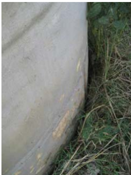
Photo-4.79 Gap between the main tower and the ground behind
