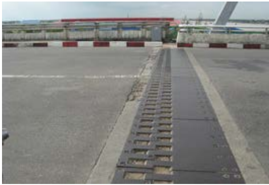
Photo-4.57 Damaged expansion joint
