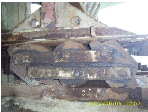
Photo-3.5 Deformed shoe of the Maubin Bridge (1)
