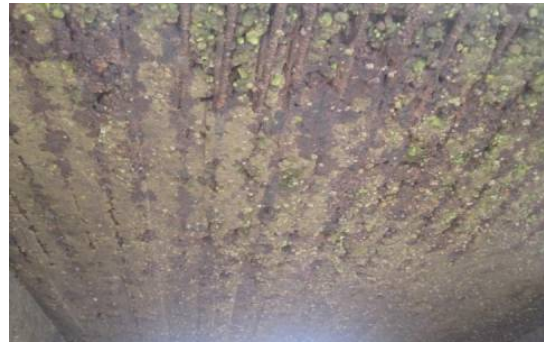
Coverless of Pile Cap bottom surface at Bayintnaung Bridge
