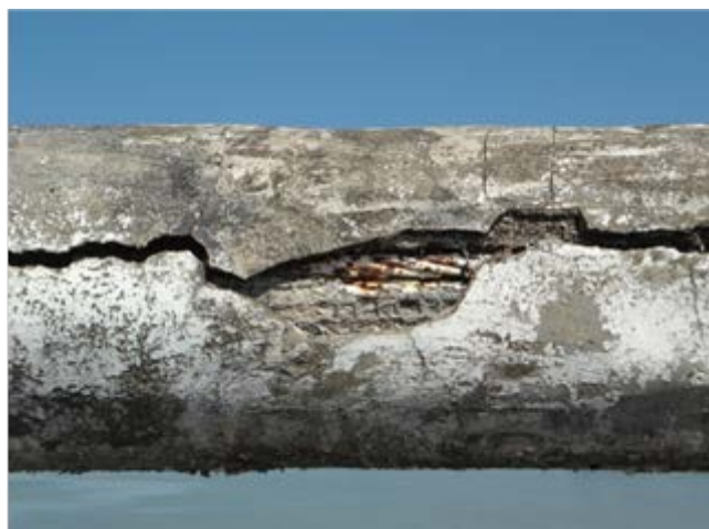
Photo—4.39 Splitting and erosion of main cable cladding
