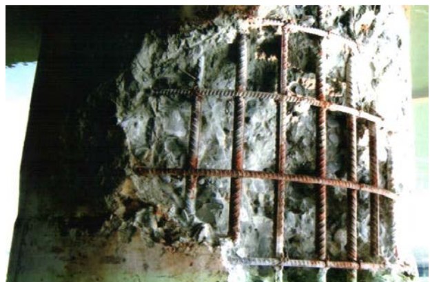
Photo-3.12 Section of poor execution at the pile top
