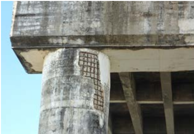
Photo-4.60 Damaged concrete pier
