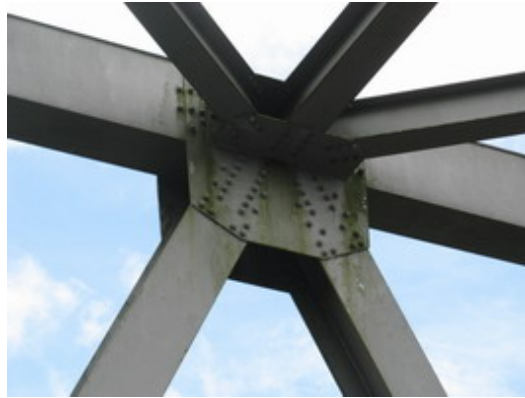
Photo—4.33 Rust at the panel point of the truss
