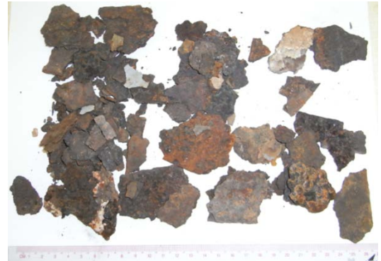
Photo-4.65 Fallen rust fragments
