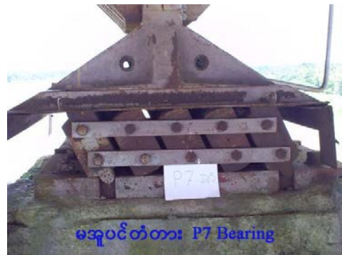
Photo-3.6 Deformed shoe of the Maubin Bridge (2)
