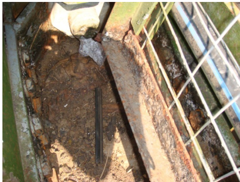
Photo-4.82 Corrosion of the hanger rope attachment
