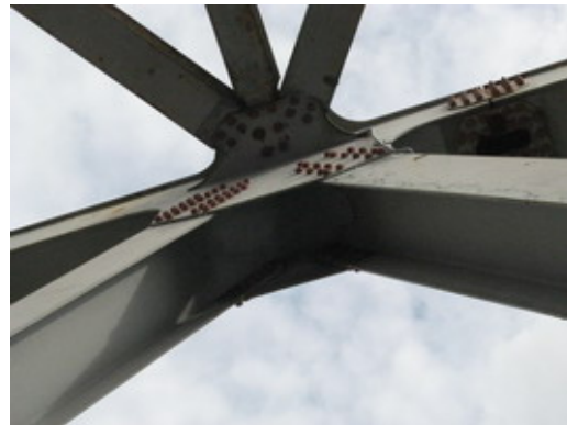
Photo-4.56 Rust of the panel point
