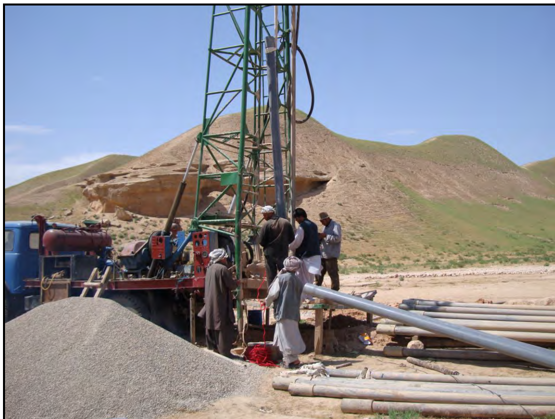
Figure 5.9. Drilling a test borehole in the Astana Valley. Photo by Engineer Hassan Saffi, DACAAR, 8 th April 2008.
