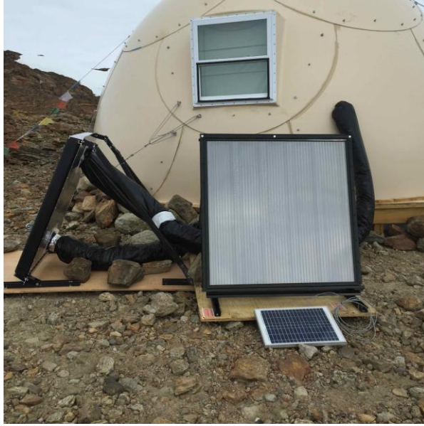
Image 6: Solar Air Heater in use for accommodation pods at Whichaway Camp
