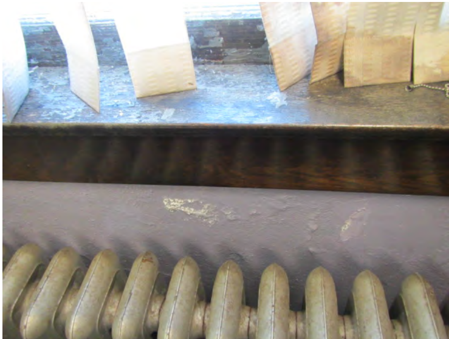
Efflorescence below first floor window underneath paint
