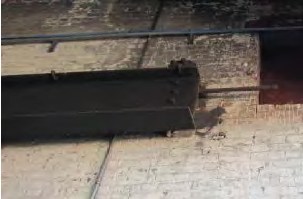
Close-up of cut beam, note uneven end
