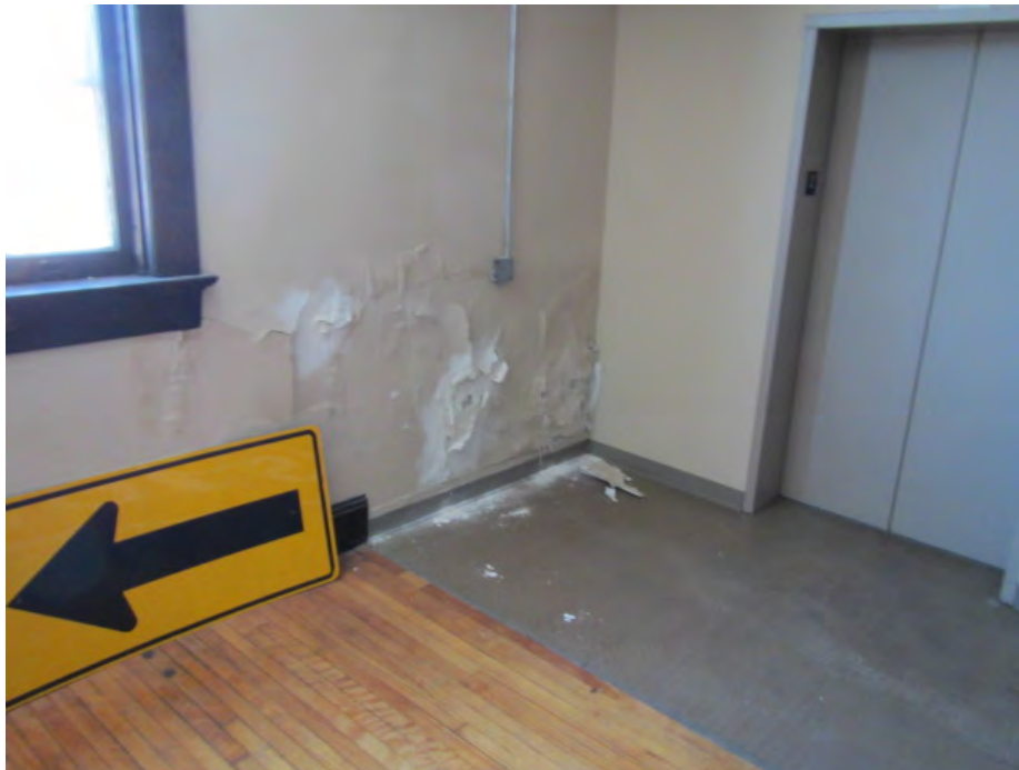
Efflorescence and peeling paint, second floor
