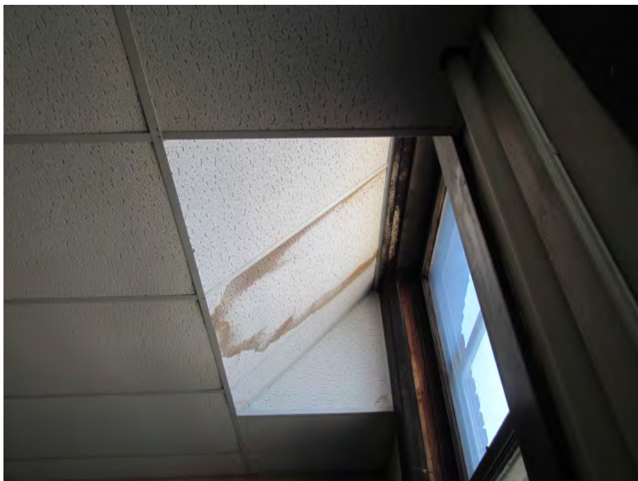
Water-damaged ceiling tile at window
