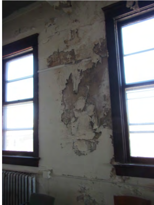
Efflorescence and peeling paint, second floor
