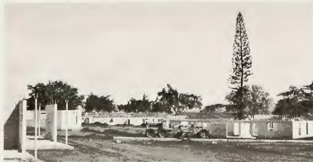
WEBB Hawaii third party building since 1964 has included home and apartment construction, such as current 1080-unit military project under a $24.9 million contract. Note how,
