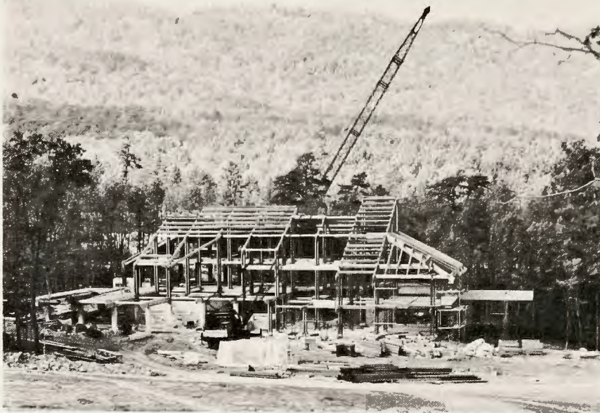
THE GOLD in "them thar hills" today is most often in the form of skiing operations, and what may appear in the photo above to be the skeleton of a mountain mining operation, is actually the partially-built ski lodge at Massanutten. Webb developers already have in place ski lifts, and machinery to produce artificial snow as an assist to nature.
