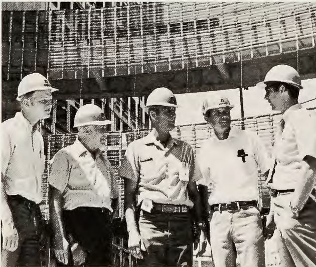
WEBB staff which "makes the job go" at Las Vegas City Hall include, from left: Chris Morgan, engineer; George Redhead, office manager; Wayne Holland, superintendent; Jim Meadows, assistant superintendent and Jim Harrison, manager of project operations.
