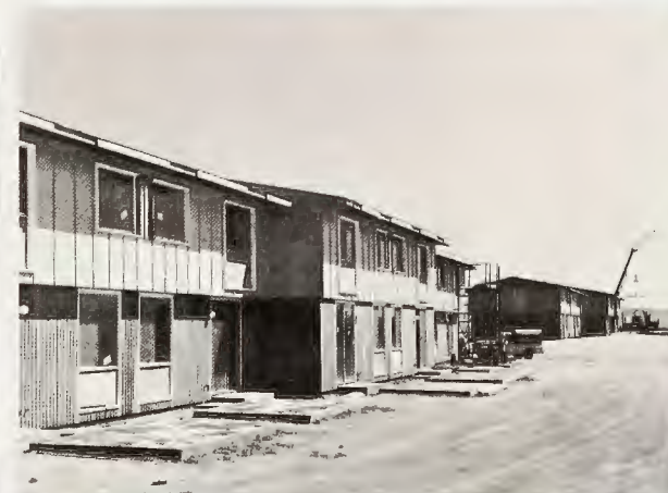
WEBB-GENERAL ELECTRIC project at George AFB, Calif. may be indicative of housing industry future. There, Webb is erecting 200 industrialized prototype units produced by G.E. in a nearby plant. Top photos show module being swung into place, while bottom photo reveals completed units, awaiting landscaping. Average apartment unit consists of 10 modules.
