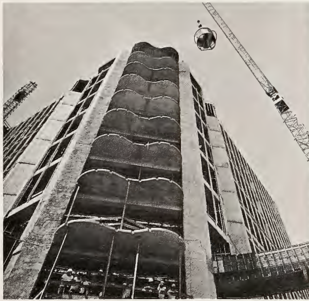
CONTINGENT of workmen, who watched entire ceremony, viewed the bucket on its way to 11th floor.
