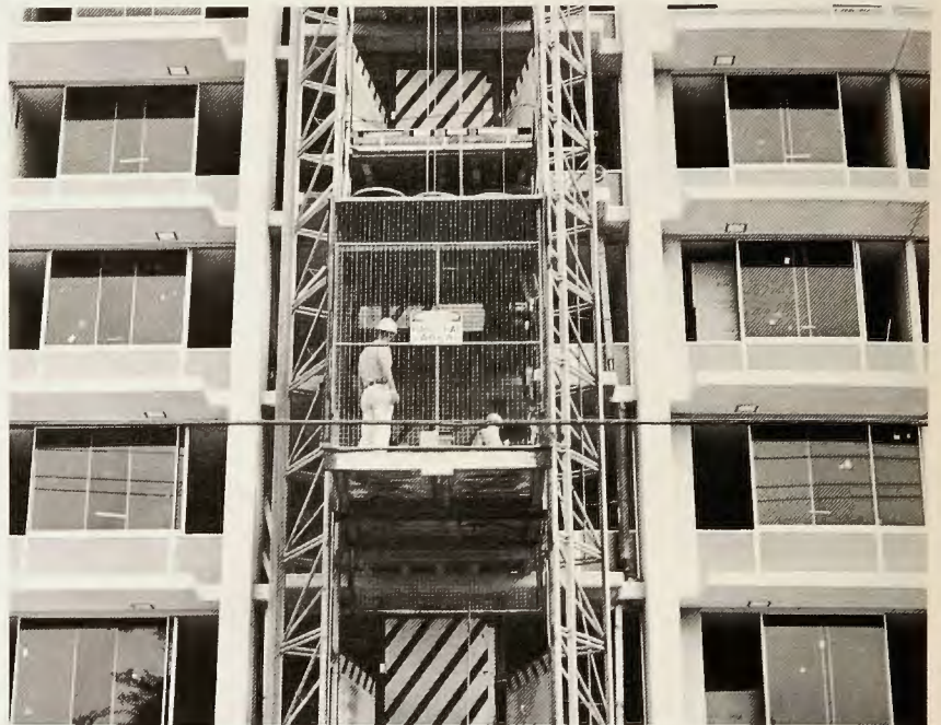
RAILINGS , painted in "loud" yellow and black to attract attention, are one of the many safety devices employed in high rise construction when materials elevator is used for passenger service as well. Shown is apartment building Webb is erecting in Phoenix for Odd Fellows-Rebekah Housing, Inc.
