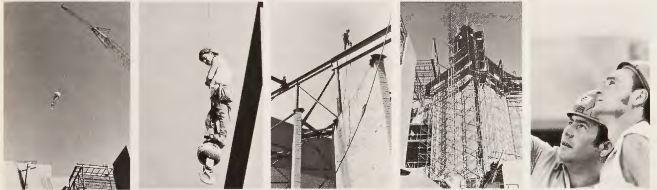
STEEL WORK , as these Phoenix Civic Plaza photos show, still requires plenty of skill and nerve.
