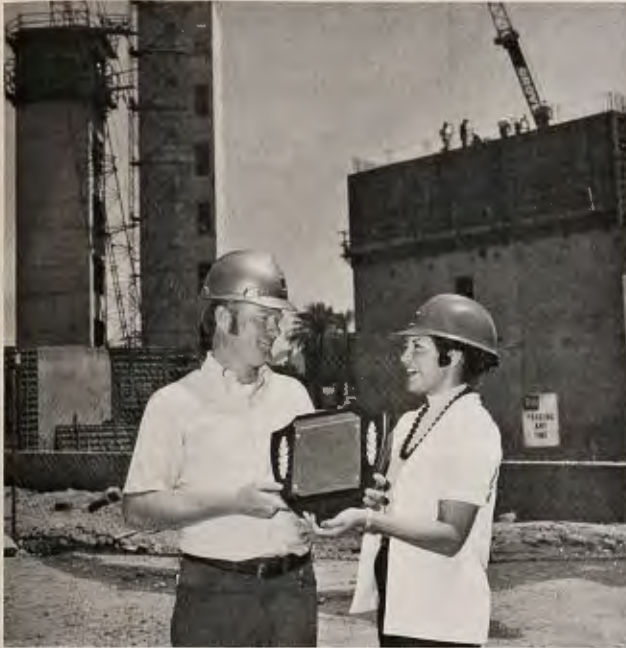
TOP MAN in May safety competition among 20 heavy construction superintendents for Webb was Jon Ancell, assigned to Arizona State University's six-story Physical Sciences Center addition. Here Ancell receives a plaque from Doreen Glantz, supervisor of loss control systems. Reasons for award, according to Jim Vay, operations manager, include installation of safety nets inside the structure's 106-foot and 98-foot elevator shafts (which extend 22-feet into the basement). Craig Hazeltine is engineer and Jim Kimball office manager of the Tempe project. SAFETY TRAINING in the area of patron protection, use of "chokesaver" for all Webb valley
