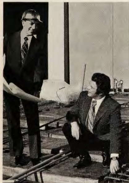
CONTRACTING group project, expanding ballroom/convention space at the firm's Sahara-Tahoe Hotel, is surveyed prior to floor pouring by John Ianni, hotel assistant general manager, left, and Tam Ryan, director of sales.
