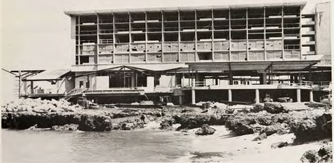
THIS PHOTO of rising Kuilima hotel reveals that rooms and public areas are taking definite shape. Shown is one of three wings of the 500-room resort, with steel in place for (from left): Kuilima
