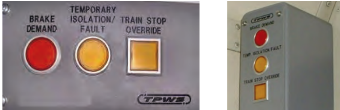
Examples of standard TPWS control panels
