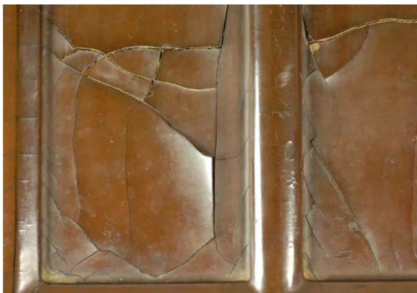
Figure 3.18.: Detail of the Chinese cabinet (F.E.7-1973) drop front inside. Extensive cracking and cupping of the lacquer coating has developed due to shrinkage of the restrained wood substrate. (Photograph by N. Schellmann, courtesy of the V&A).
