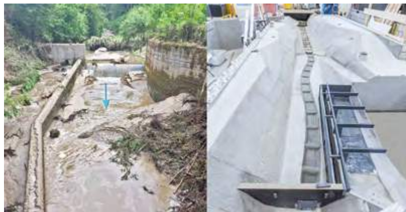
↓ Fig. 1, left: Clogged flow diversion structure after a flood event in June 2015; right: Hydraulic model at a scale of 1:15. View against flow direction.
