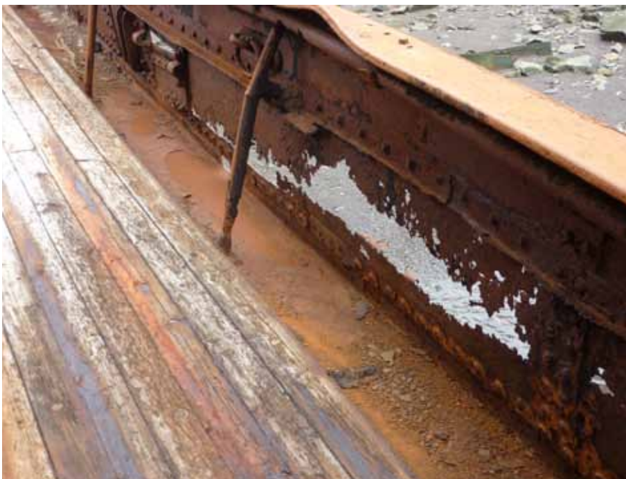
Corrosion on the starboard bulwark of Dias
