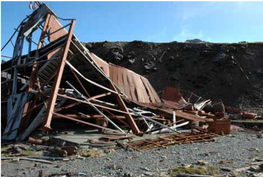
The collapsed Store No. 3 at Leith Harbour. Substantial steel frame buildings can collapse.
