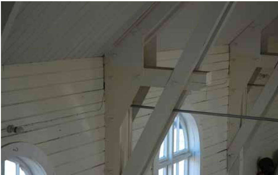
Strengthening of the roof trusses with steel plates carried out in the last few years. The work was apparently carried out by Tim Carr, the Museum Curator.
