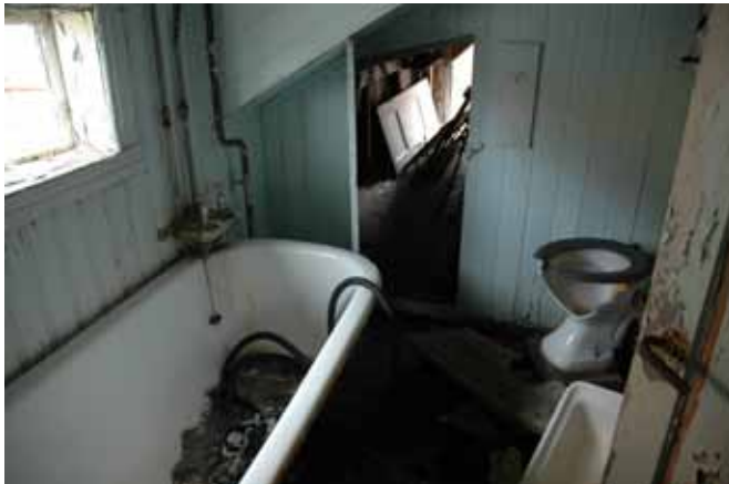
First floor bathroom in building No. 16. Possibly the bath used by Shackleton!
