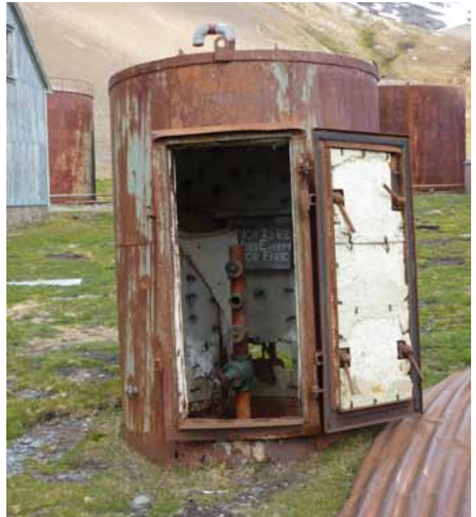
One of the fire hydrant points around the site at Stromness
