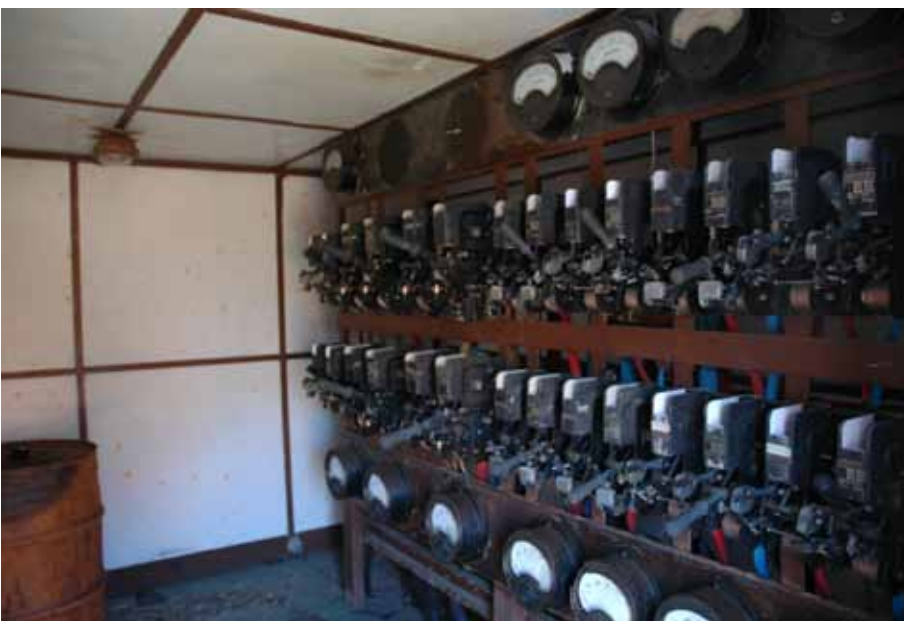
One of several switch rooms, this one in building No. 20 at Leith
