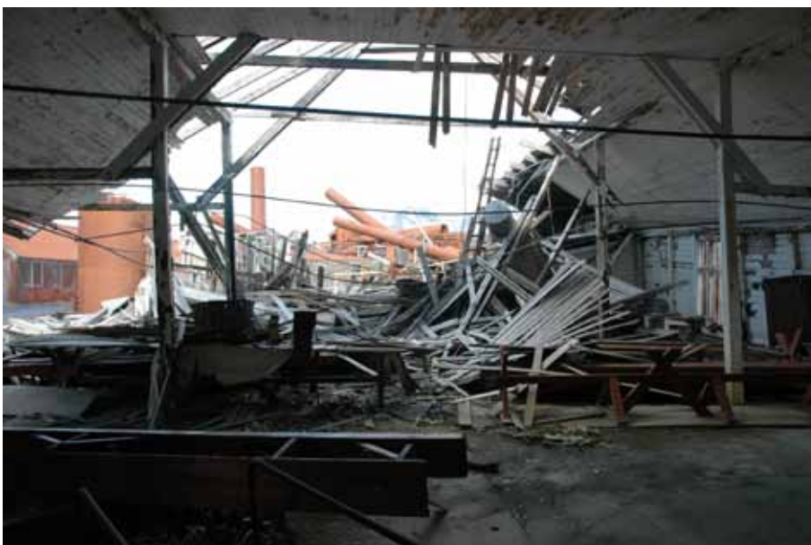
The collapsed end of the Mess Building at Husvik
