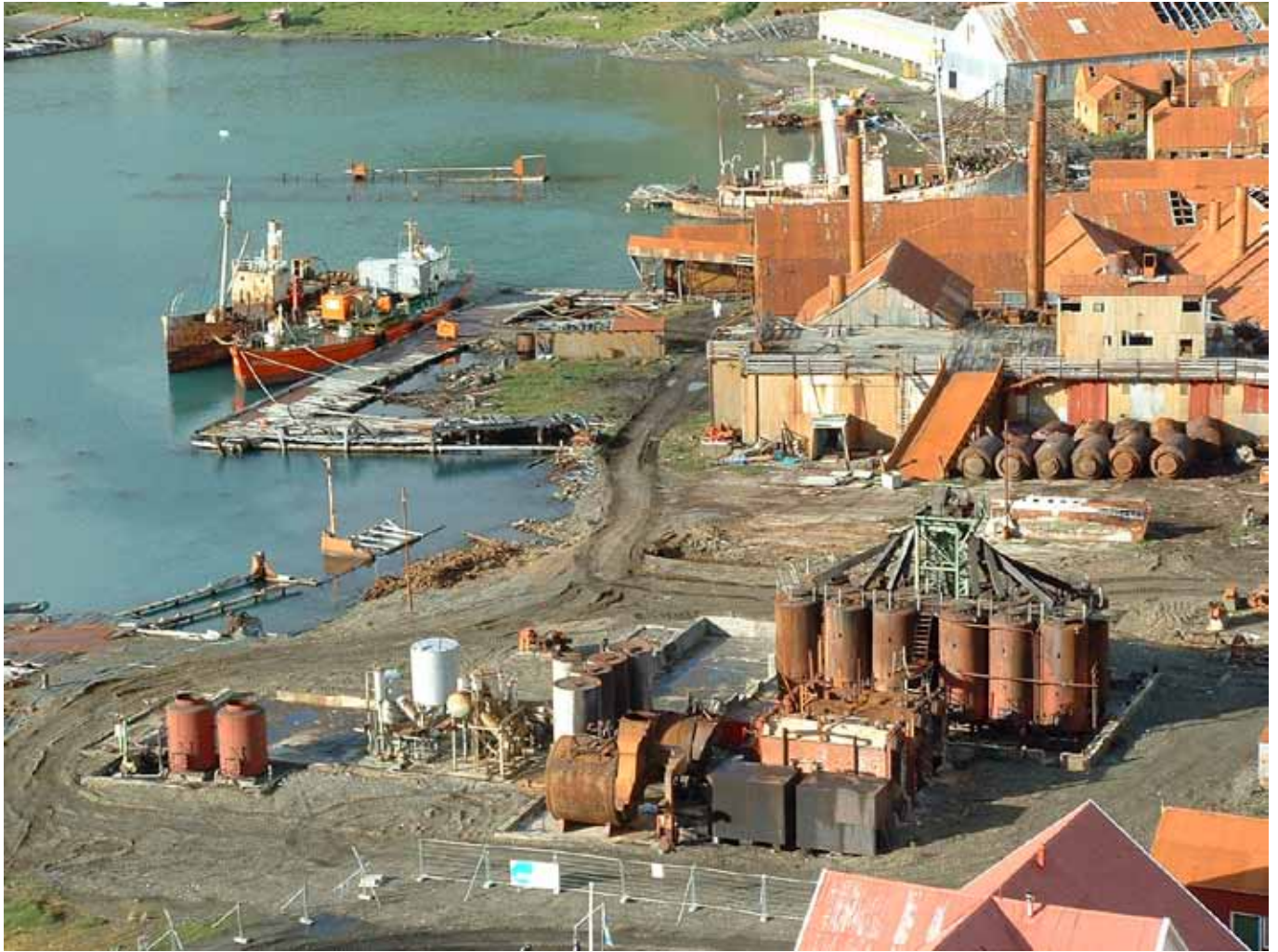
A view across the site in 2003/04. The Boiler House and Blubber Cookery are already demolished but work has not yet started on the Meat Cookery and Guano Plant.
