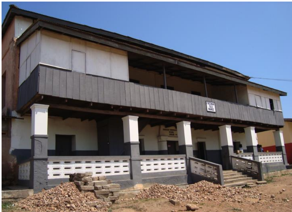
Figure 18. Methodist Mission, Rev. George Wrigley, Rev. Thomas Birch Freeman, and Henry Barnes, c. 1839-40, rammed earth and timber, Anomabo, Ghana. 2009 (author's photo).
