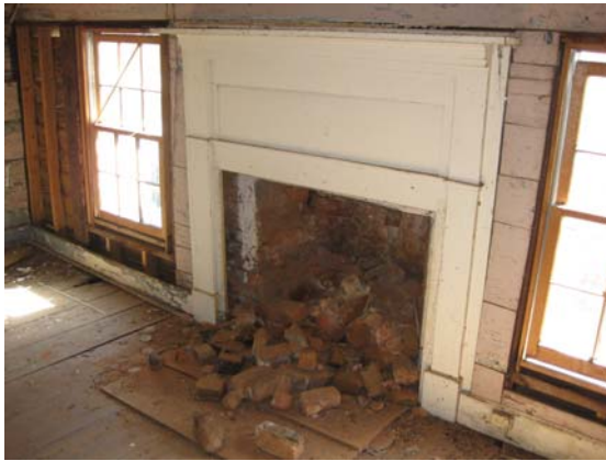
Second floor, note collapse of firebox
