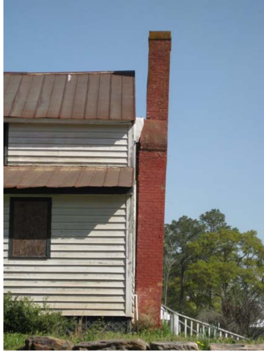
6. Partial South Elevation, Note opening at wall and out-of-plumb chimney condition
