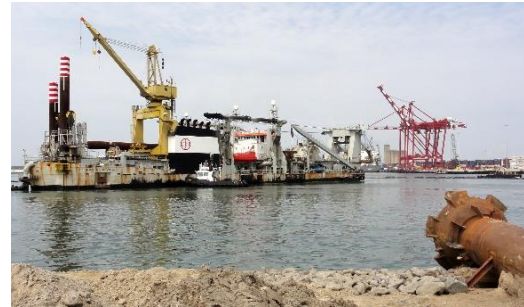
Capital dredging and reclamation for the second phase of the Eastern Extension of the Port of Pointe-Noire (Congo)
