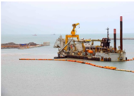
Quay wall construction for the extension of the harbour of Takoradi – CSD Ibn Battuta (Ghana)
