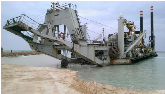
Capital dredging works for the access channel and port basin of the green port of Kuryk - CSD Vesalius (Kazakhstan)
