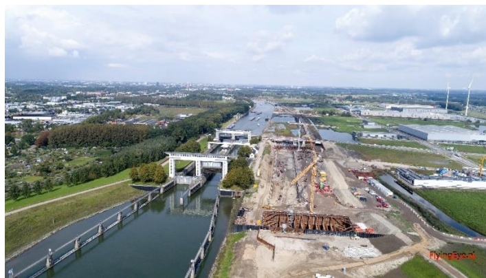
Construction of a third lock for the Beatrix Lock complex (the Netherlands)
