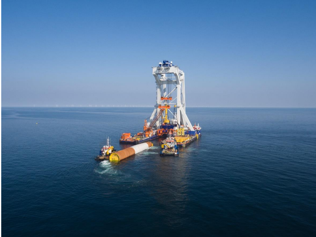
Van Oord's top duo Aeolus and Svanen have successfully completed work on the Walney Extension offshore wind farm
