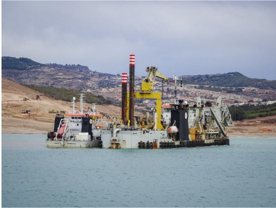
Construction of new container terminal in the Nador West Med Port, CSD Zheng He & SHB LAigle (Morocco)
