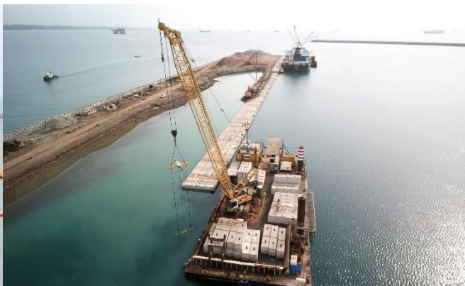
Quay wall construction for the extension of the harbour of Takoradi (Ghana)
