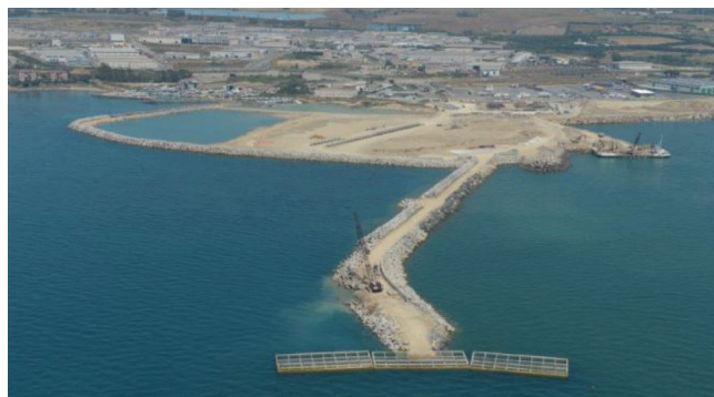
Port of Civitavecchia: Ferry Dock – Construction of Lee Breakwater with caissons REWEC 3 type B
