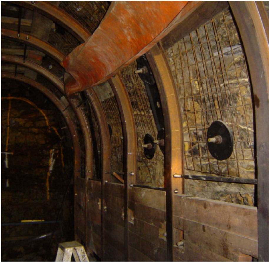
Figure 7. Type 4 supports – steel mesh with rock anchor bars, curved steel sets bolted together and timber lagging in between
