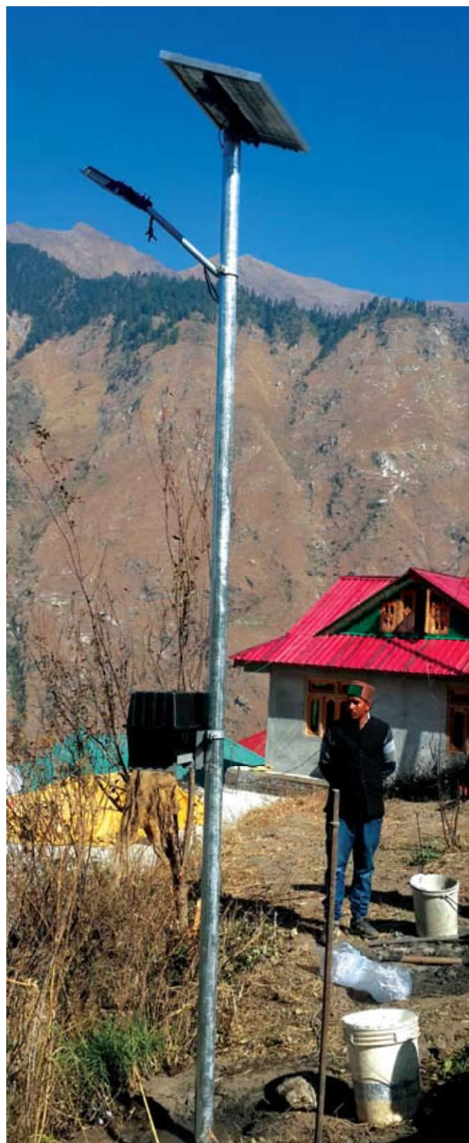
Solar PV street lights installed in Himachal Pradesh
