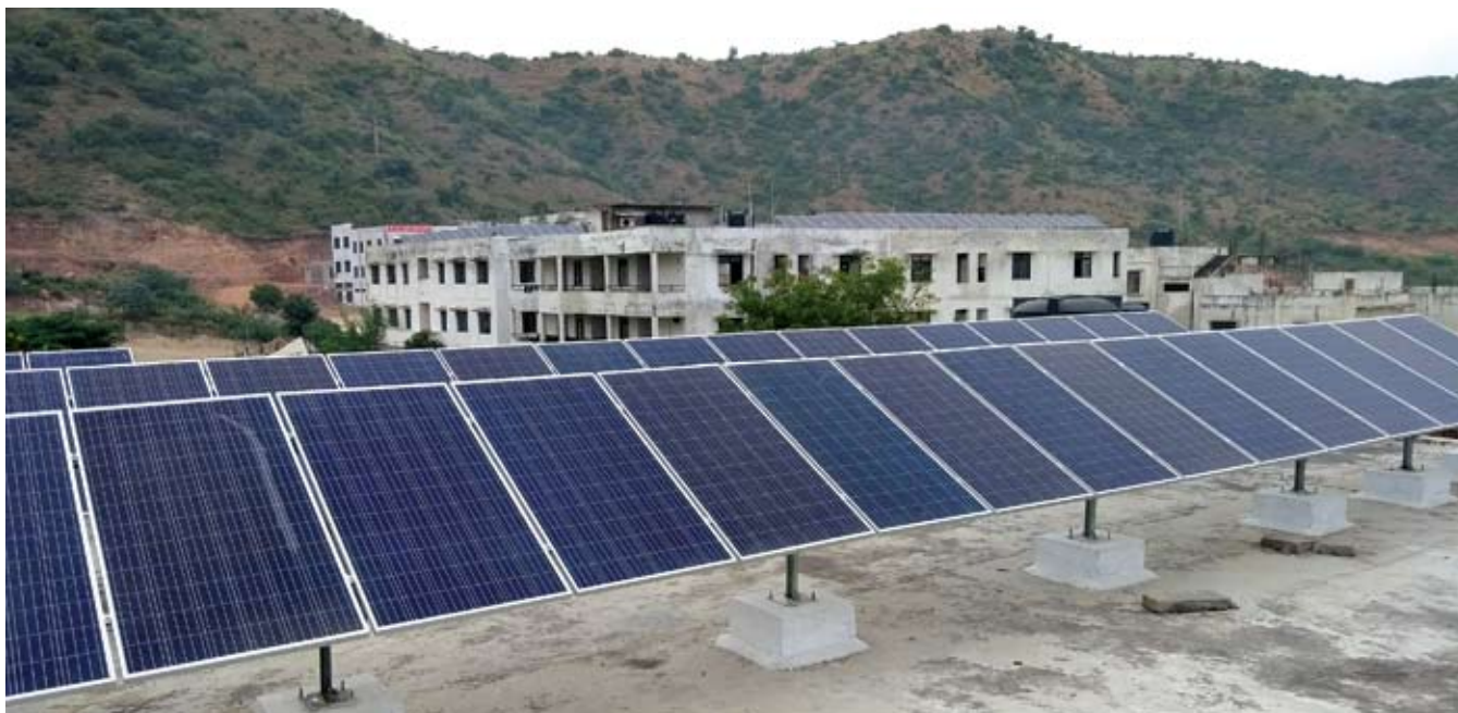
Grid connected solar rooftop plants of 300 kWp installed by SECI at SS College of Engineering, Udaipur, Rajasthan
