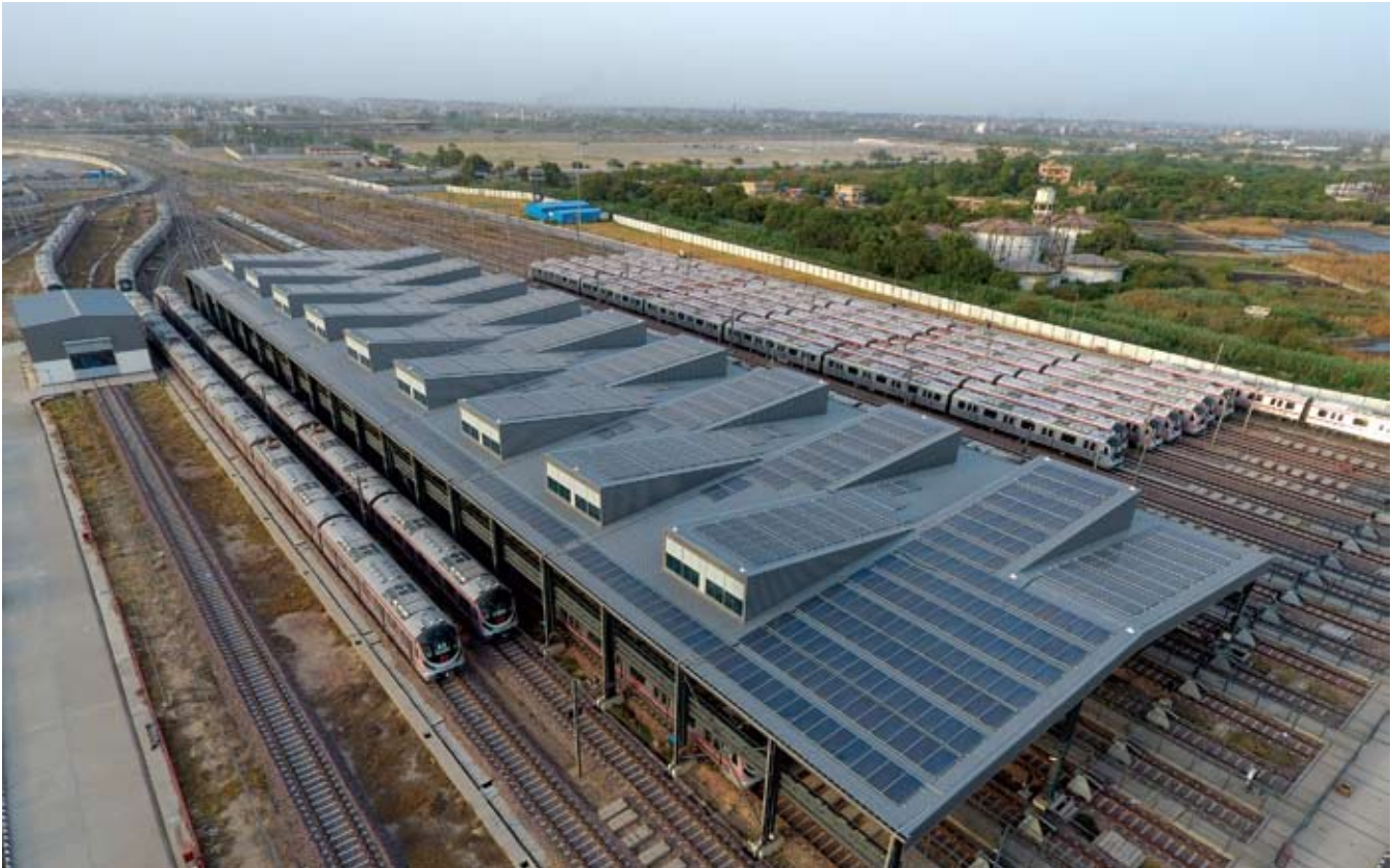
Grid connected solar rooftop plants of 387 kWp installed at Mukundpur Metro Station of Delhi Metro Rail Corporation Ltd.
