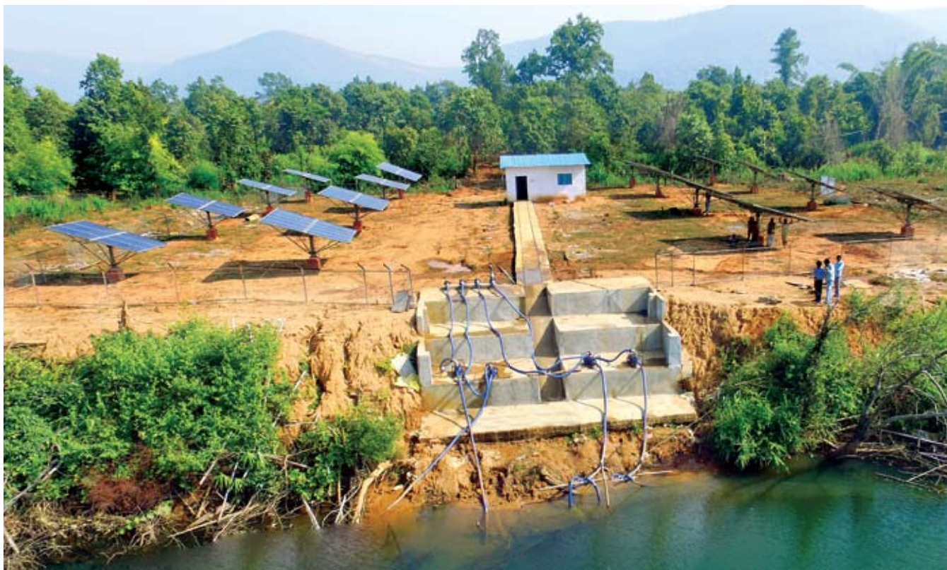
Community Solar Pump Systems installed at Kulhadighat Distt. Gariyabandh, Chhattisgarh
