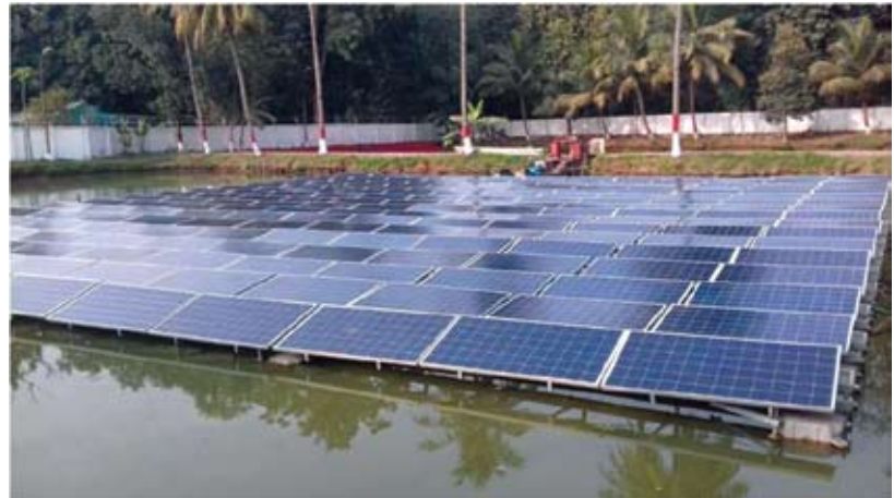
Installation of 60kWp Floating Pond Top Solar Power Plant at Hon'ble Governor House in Bihar
