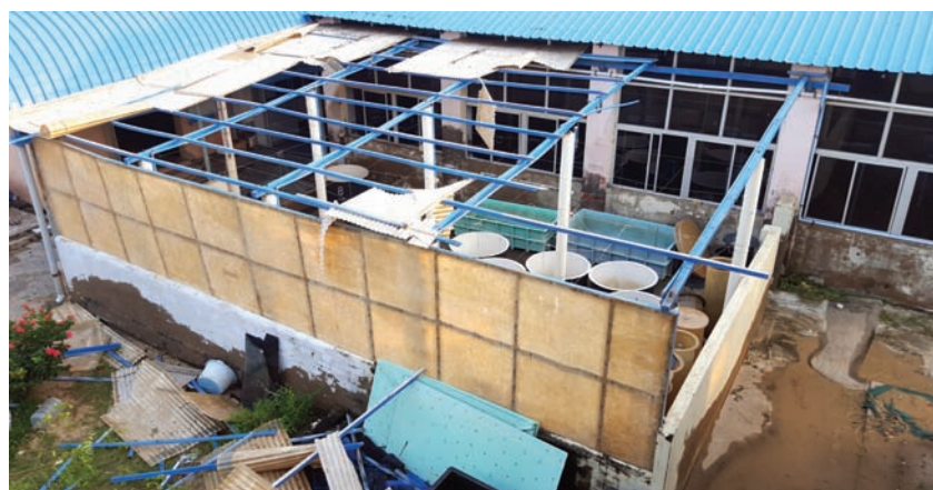
Kovalam lab damaged by Cyclone Vardah
