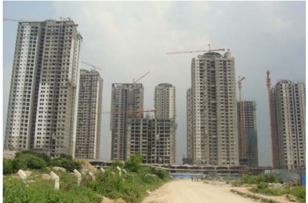
The Real estate Project (Lanco Hills) towering upto 33 floors in Manikonda, a sought after location for real estate growth
