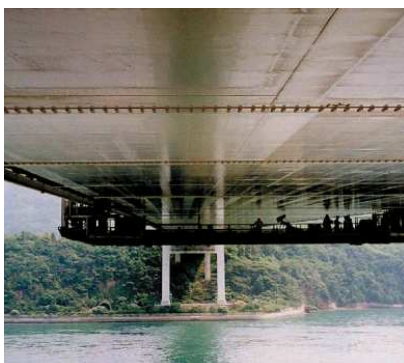
Movable maintenance platform
