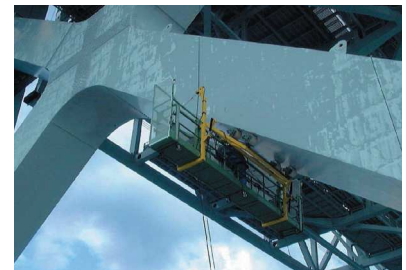
For diagonal and horizontal member (work on under side of diagonal member)
