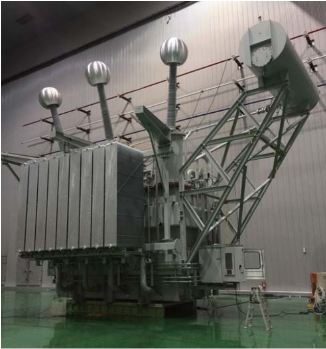
6 345-kV/265-MVA power plant transformer
