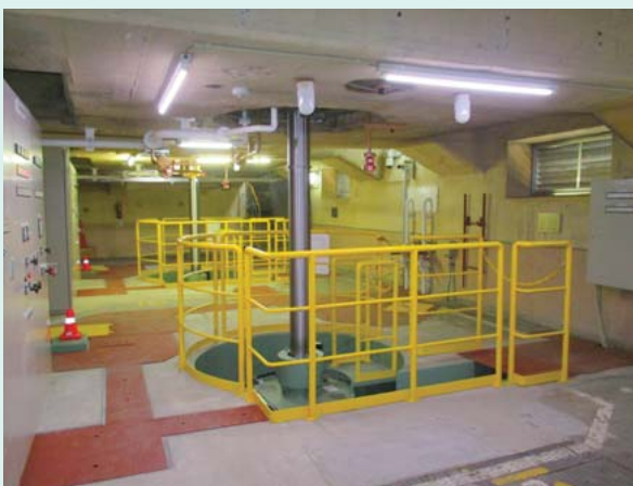
3 Kakinosawa Power Plant generator room (top) and turbine room (bottom)
