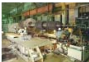
Staff from Okinawa Plant Kogyo Company, Incorporated disassemble a turbine at Makiminato Thermal Power Plant for a regular inspection.
