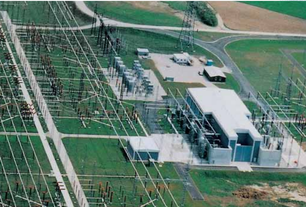
Fig. 2-3: Back-to-back converter Station Vienna Southeast
