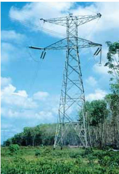
Fig. 5.6.1-1: DC transmission line (bipolar tower 300-kV link)
