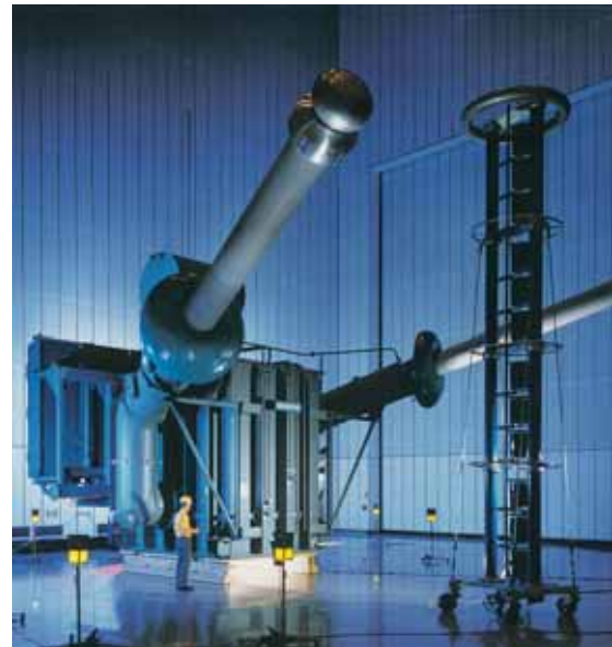
Fig. 5.3-1: Oil-insulated smoothing reactor – Three Gorges project
