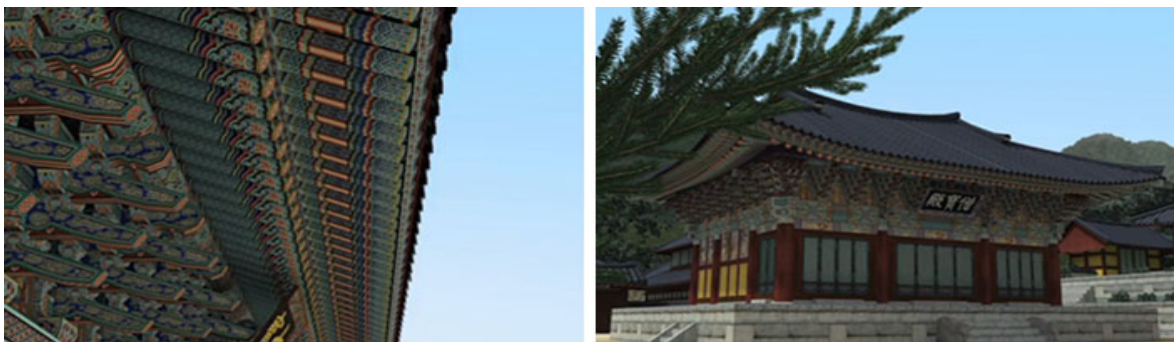
Figure 46: Bracket systems and double rafters (left) and the Sungbojern (right) from my graphic images
