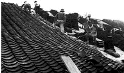
27) Tiling on the roof. Clay tiles baked at a high temperature and used as materials for covering a roof.
