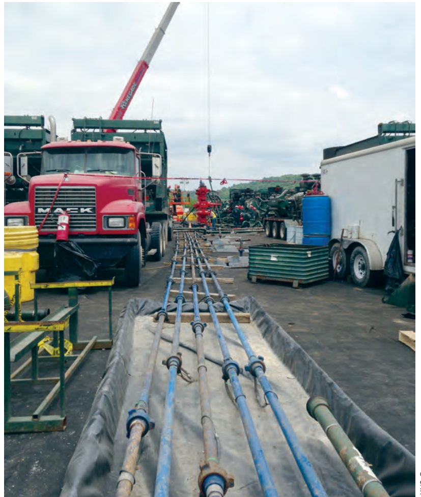
Completion equipment at a gas well.
