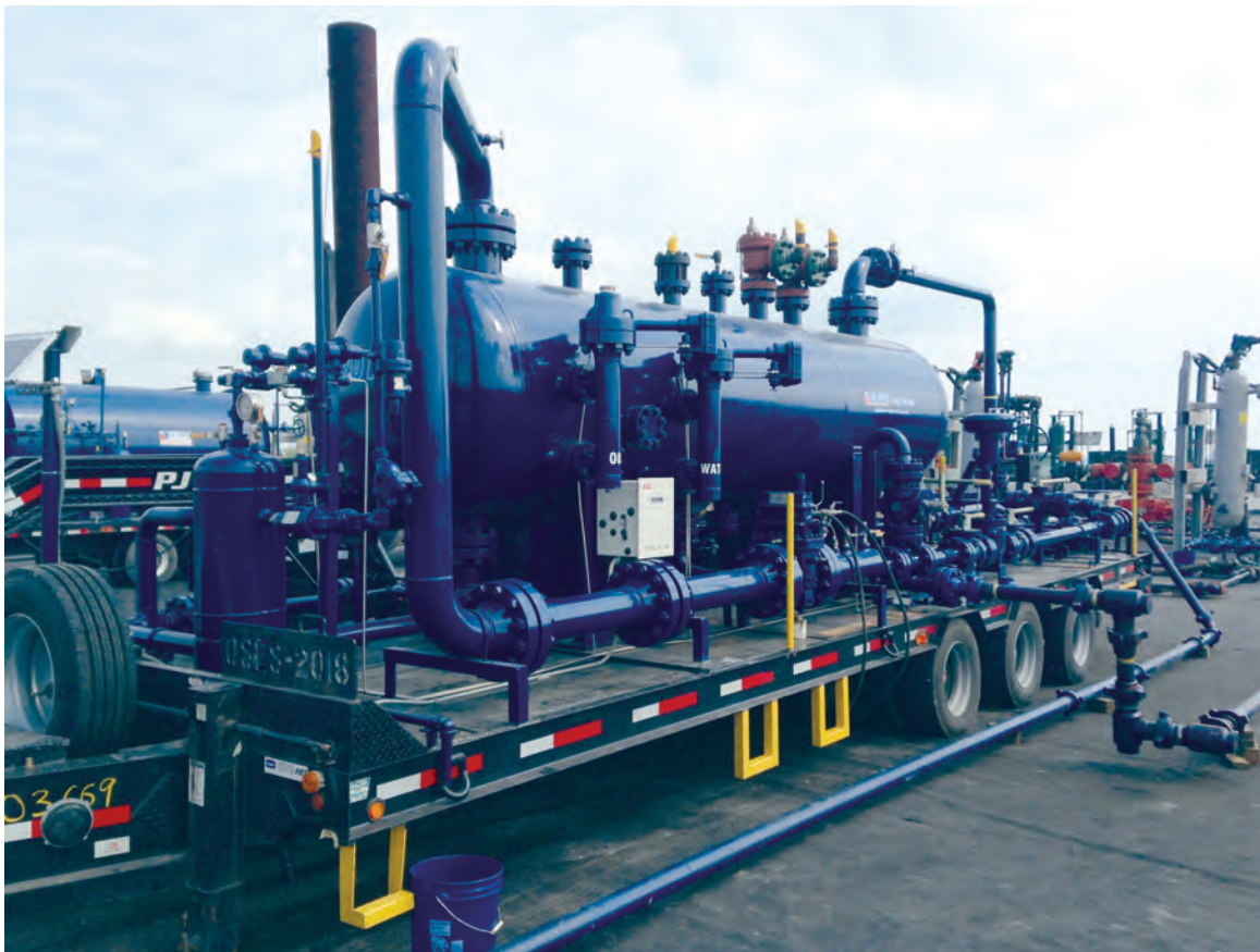
Equipment at a gas well.
