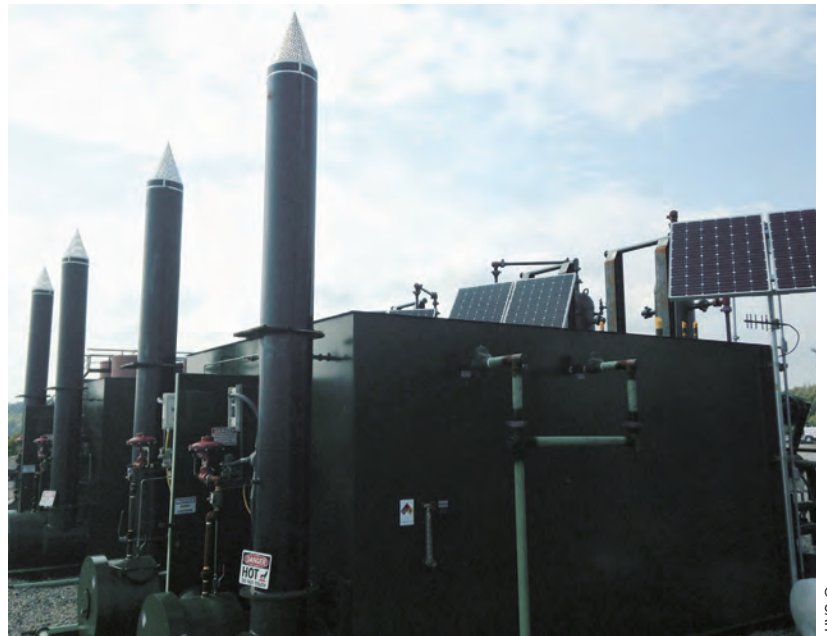
Equipment at a gas well.
