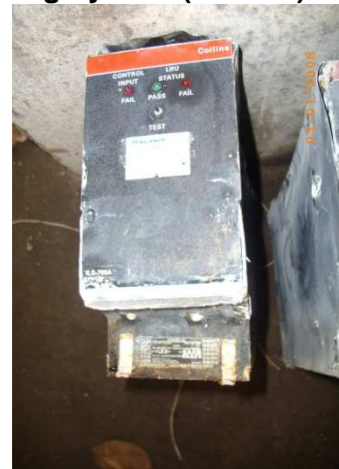
Range Instrument Landing System (S/N 852)
