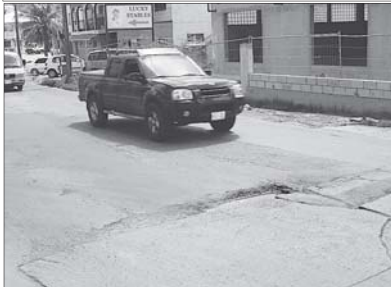
"If you are not careful, it can swallow your car!" This was how one driver described his encounter with the deep pothole on Welfare Road opposite Daily Extra Supermarket. Drivers are appealing to Public Works Commissioner Theo Heyliger to start patching the island's roads, which are becoming more and more riddled with potholes every day, as soon as possible. The Welfare Road "ravine" is also a traffic hazard, according to drivers, because many of them swerve to prevent their vehicle from plunging into it. (John Halley photo taken on Tuesday, July 10.)
