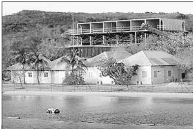
The first outlines of what's going to be the Hyatt Resort in Curaçao are rising behind Barbara Beach. The 350-room resort extends from the beach some hundred metres to the seacoast in the direction of Fuikbaai. What was used as beach-bar before is now the construction site hut, "the most beautiful in the world," jokes supervisor Raul Reinren. The developer is Geveke Development, a branch of the Dutch Vervat Group.
