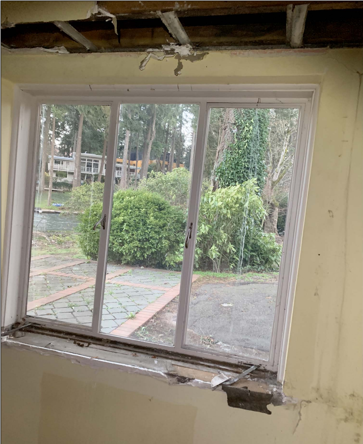
Photo 8 of 15: Failing structure and window
