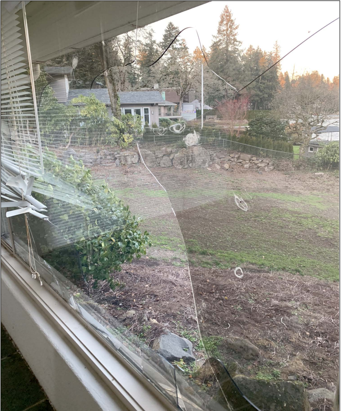
Photo 10 of 15: Broken bay window and landscaping
