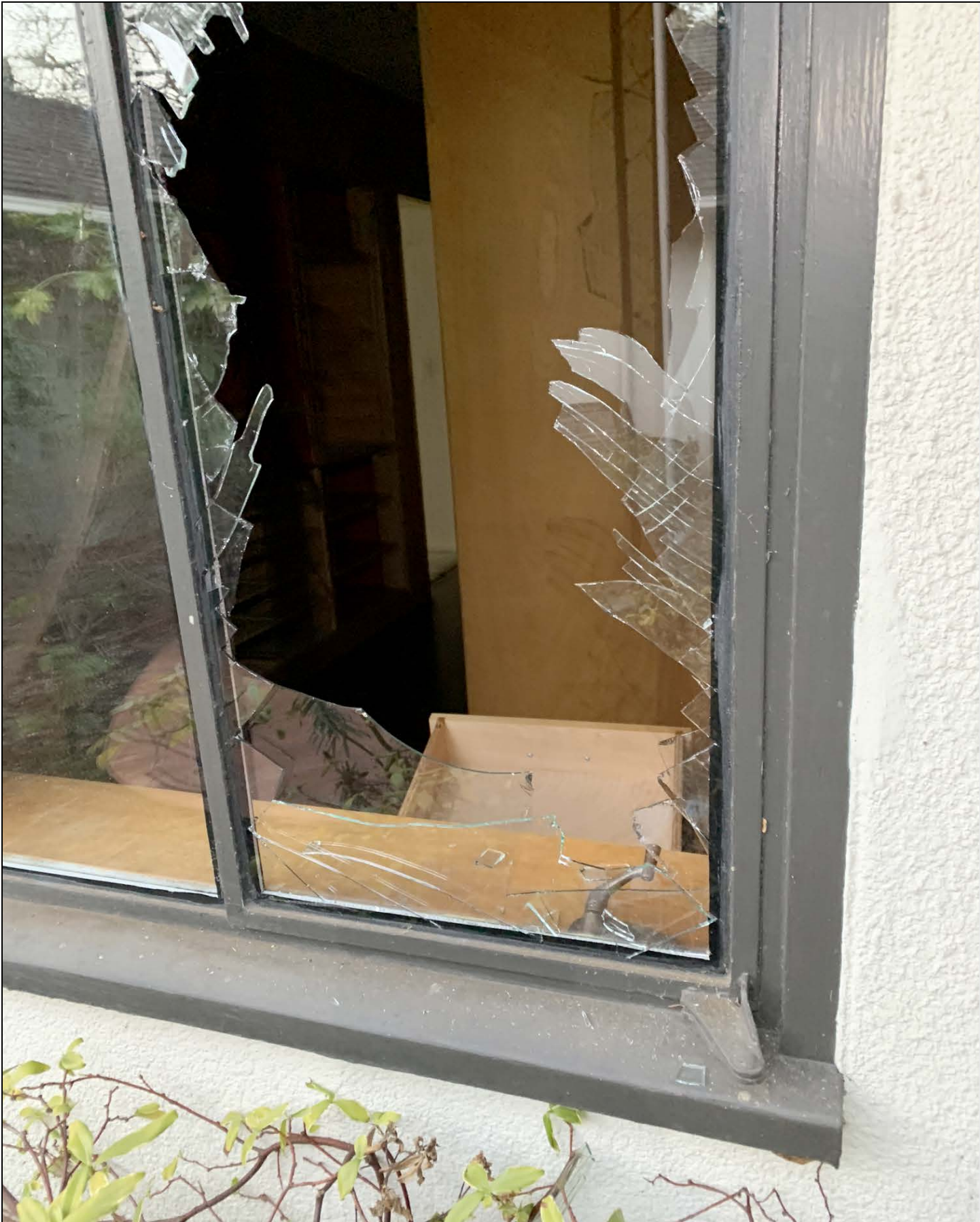
Photo 11 of 15: Collapsing and broken easement window
