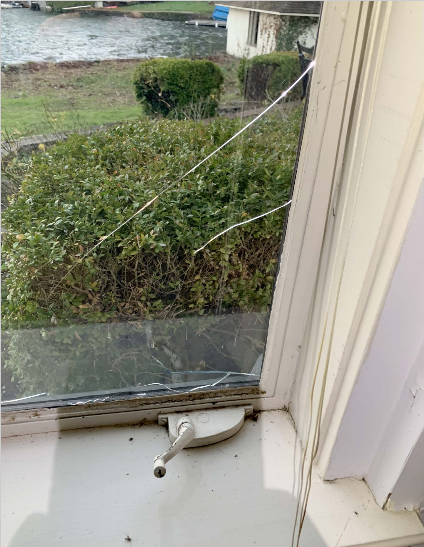
Photo 9 of 15: Collapsing and broken easement window
