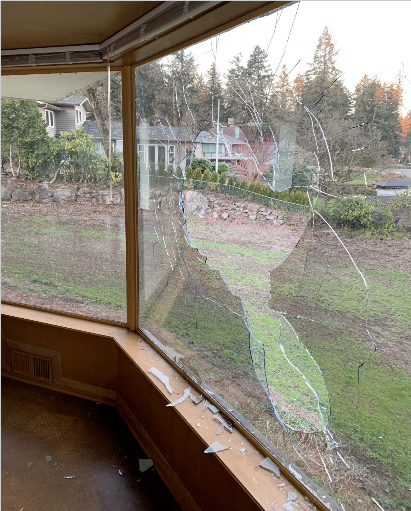
Photo 5 of 15: Broken bay window and lack of landscaping
