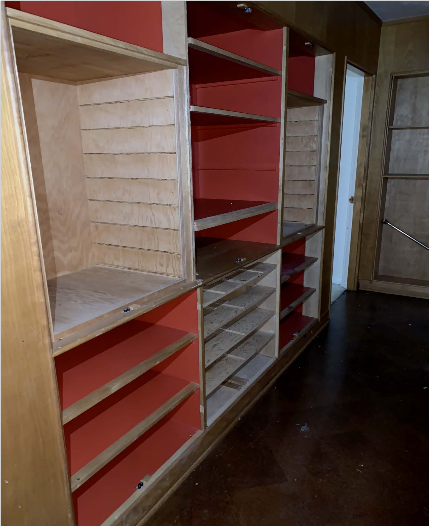
Photo 4 of 15: Stripped fixtures
