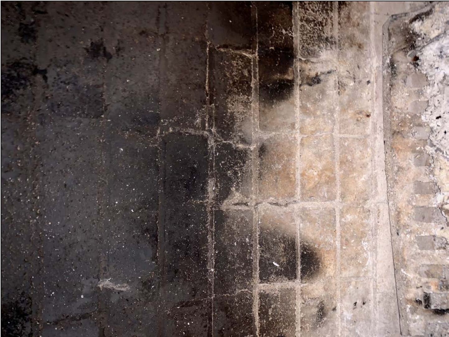
Photo 13 of 15: Destroyed/failing brick
