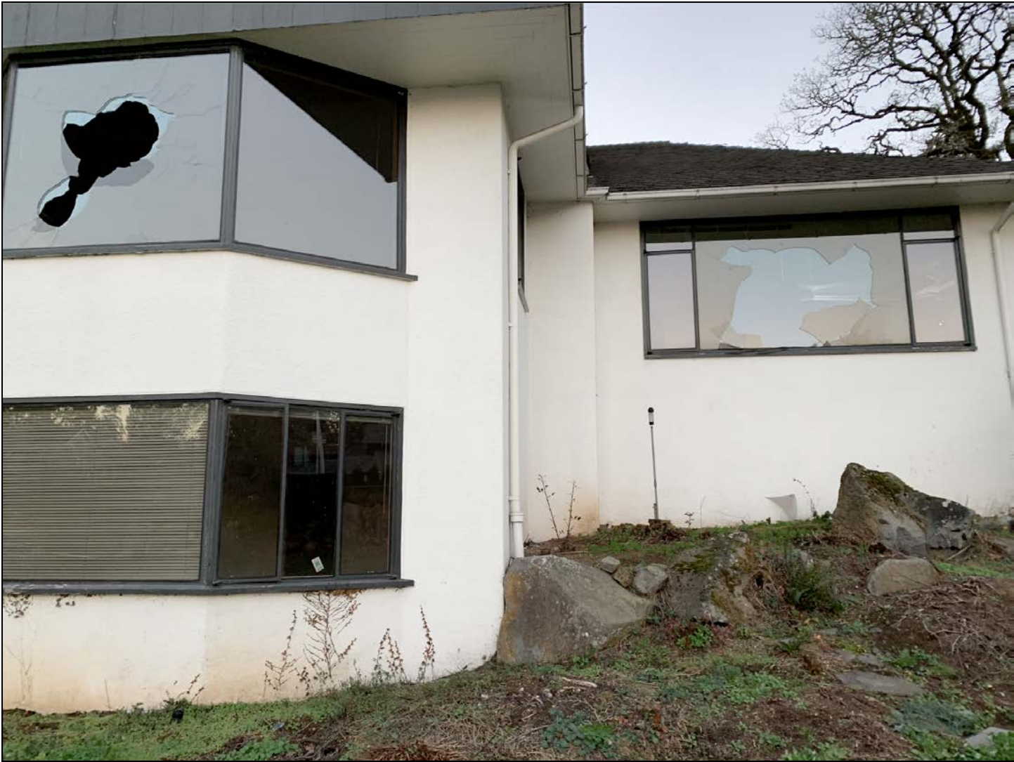
Photo 7 of 15: Exterior, broken windows; landscaping
