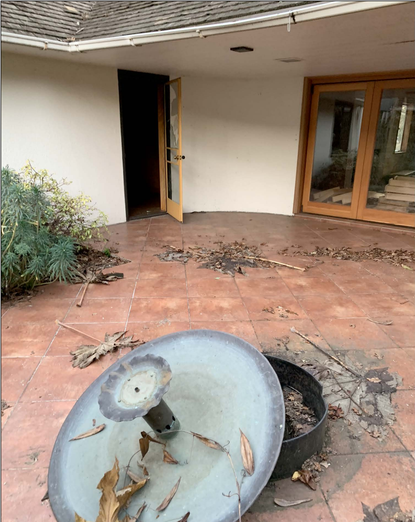
Photo 2 of 15: Courtyard and collapsing roof
