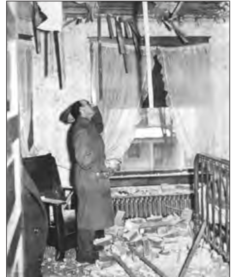
Toppled chimneys were common in Anna, Ohio, from the March 2 and March 9, 1937, earthquakes. In this home, the chimney crashed through the ceiling, scattering bricks in a bedroom. Fortunately, no serious injuries resulted from these earthquakes.
