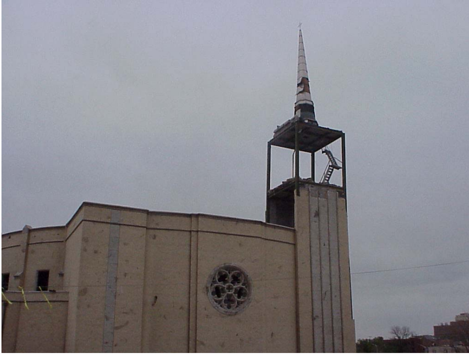
Figure A11. Calvary Temple Church steeple failure and impact markings on brickwork.
