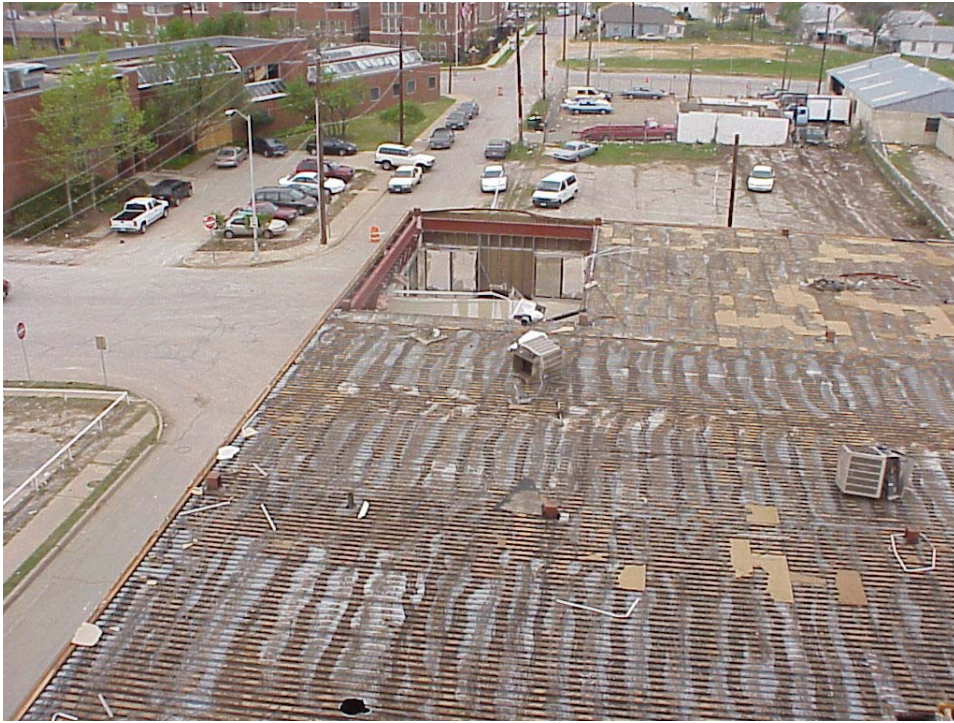
Figure A17. Failure of roofing and corner structure 933 W Weatherford.
