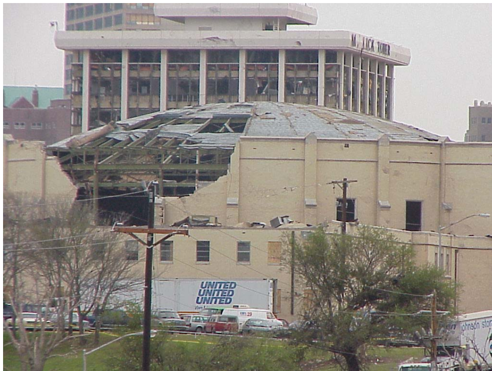
Figure A12. Western side of Calvary Temple Church with Mallick tower beyond.
