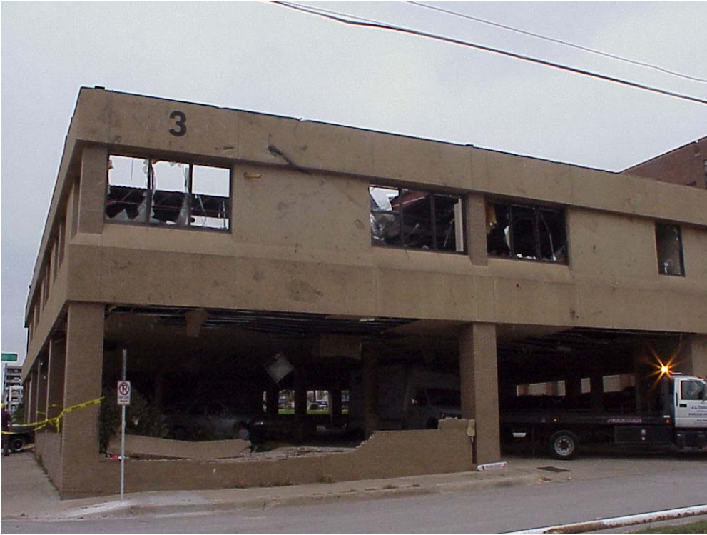
Figure A15. Southwest face of 933 W Weatherford showing failure of roof corner.
