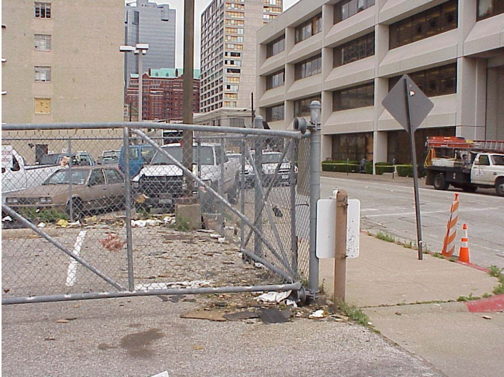
Figure A23. Bent GI gate on 2 nd Street adjacent to Hunter Plaza, bent towards north.
