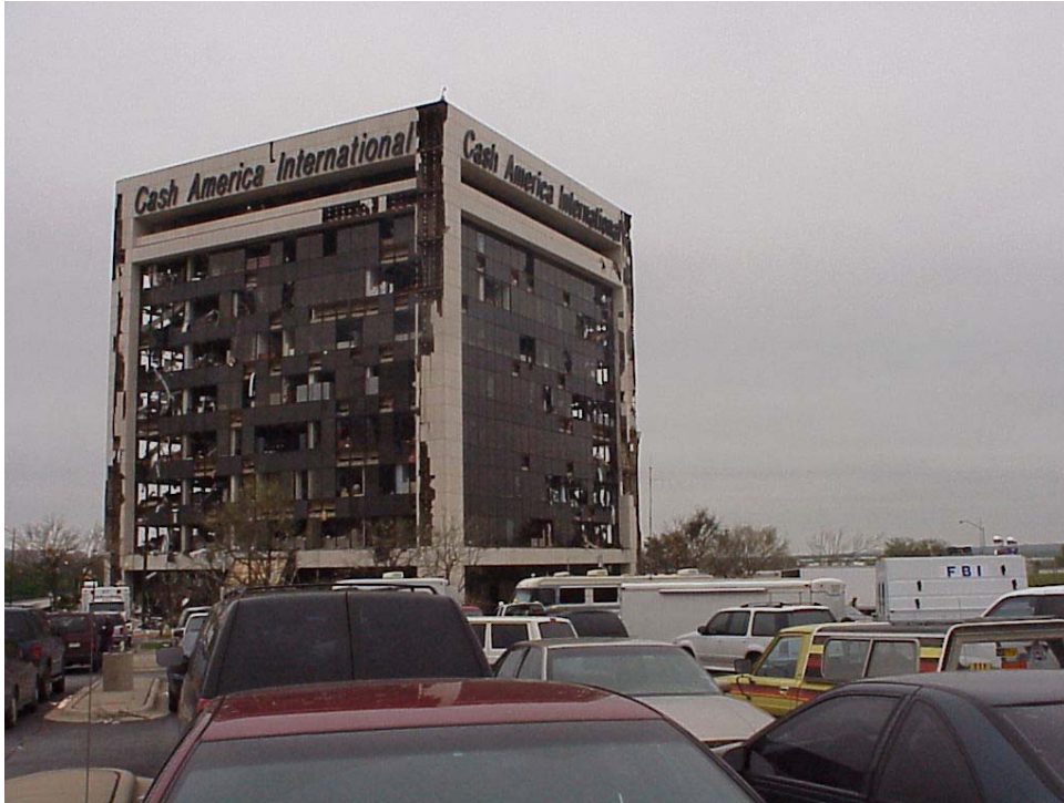
Figure A7. Southwest and northeast faces of Cash America building, showing wind damage in corner regions.
