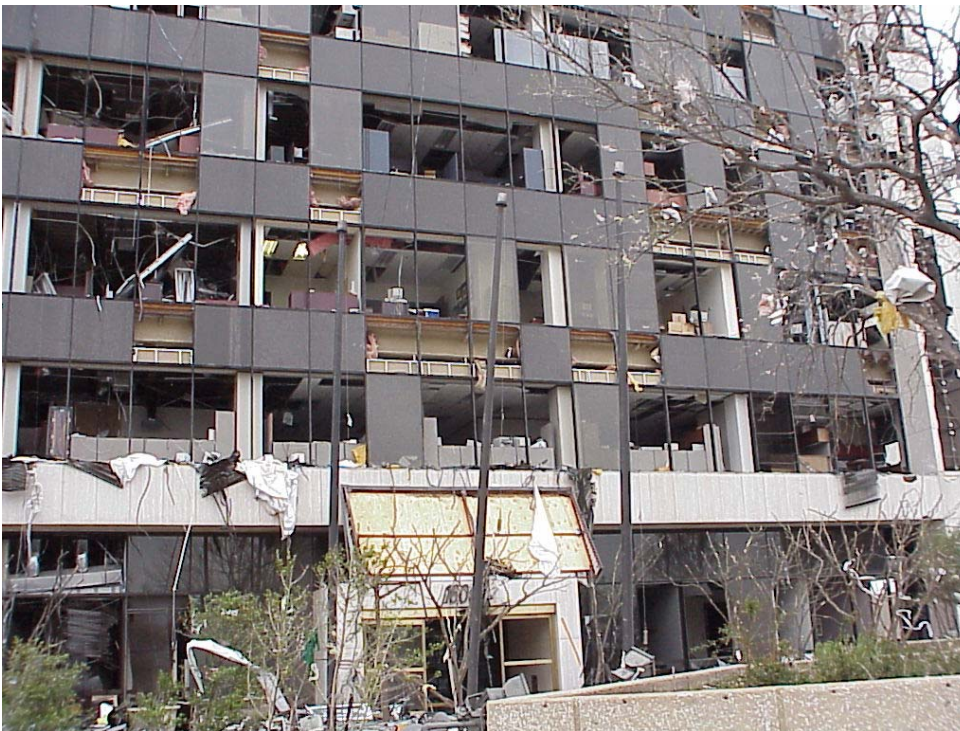
Figure A8. Southeast face of Cash America building showing uplift failure of entrance canopy.
