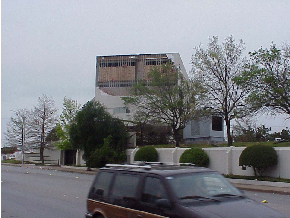
Figure A9. EIFS wall construction failure on northwest face of Education Employees Credit Union.
