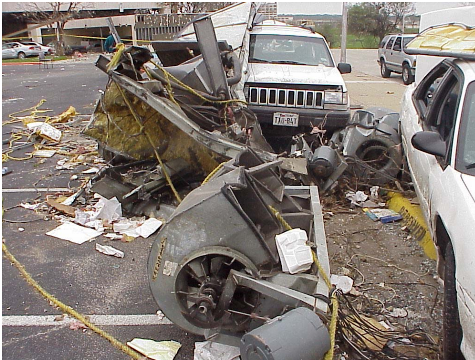
Figure A14. Air-conditioning equipment from the roof of Calvary Temple Church in W 5 th Street.
