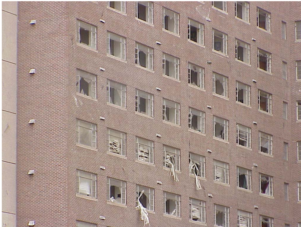
Figure A.24 Window breakage at Hunter Plaza, south facing interior of U-shaped plan.
