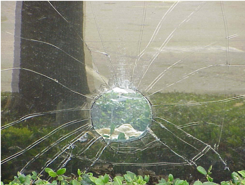
Figure A20. Impact fracture on outer lite of insulating glass unit on the ground floor of INSpire Insurance Building, southwest façade.
