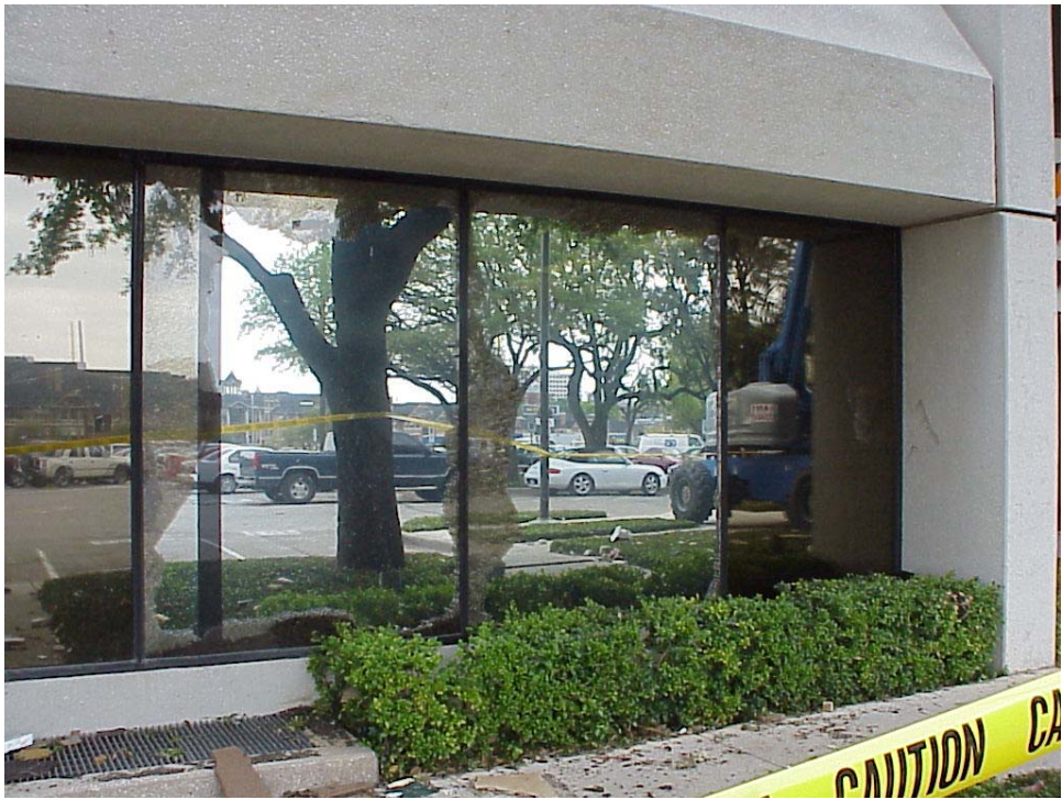
Figure A22. Broken outer lites of insulating glass units on ground floor of INSpire Insurance Building, southwest façade.
