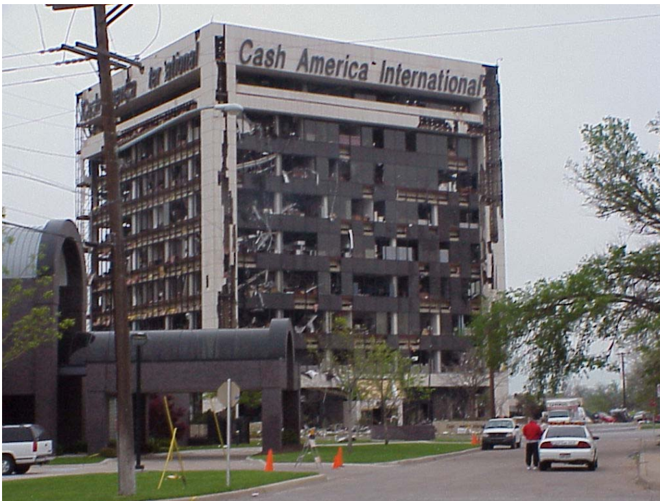
Figure A6. Southwest and southeast faces of Cash America International building, showing internal debris piled up at the south corner.
