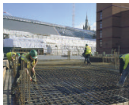
Fig 4 Construction underway of the new studios (2006) with St Pancras EuroStar Railway Terminus in background. Image reproduced with kind permission of the British Library Board.
