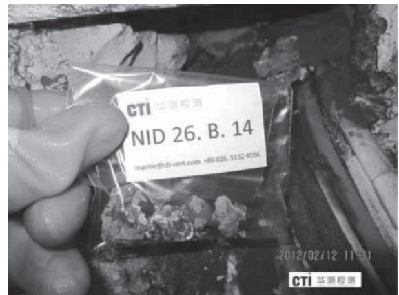
Picture: Cable penetration detected containing asbestos from newbuilding ship
