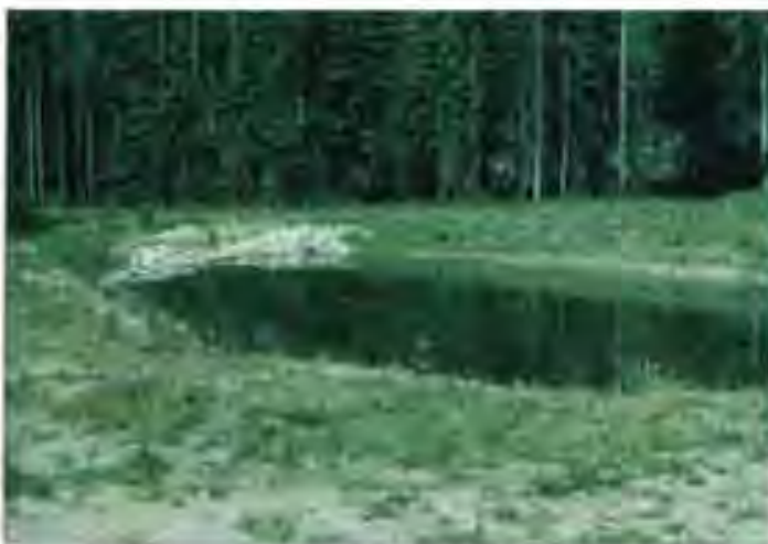
DRAINAGE IMPROVEMENTS TO LITTLE HOPEFUL CREEK IN CONJUNCTION WITH GOLF COURSE CONSTRUCTION.
