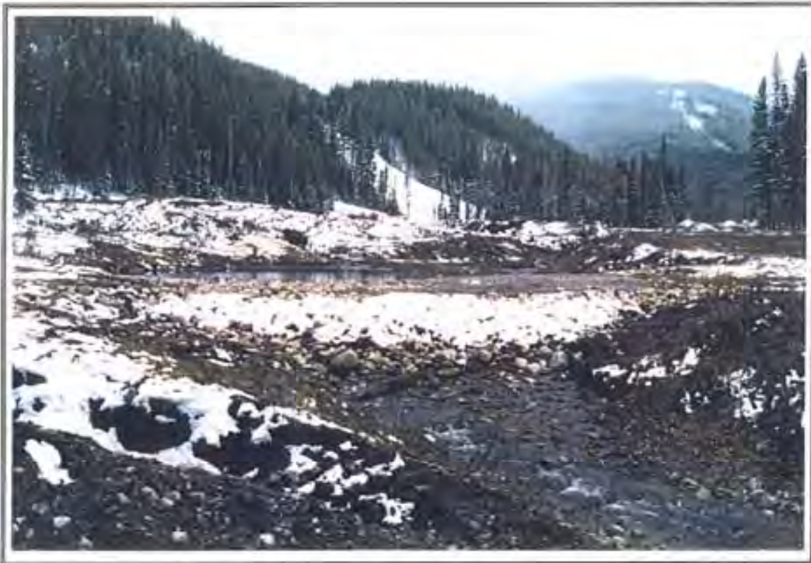
Photo 8 Settling ponds on Little Hopeful Creek (Reach 1/2 break) May 8, 1996.
