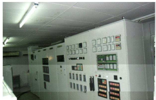
New equipment installed by NAWEC during 2011
