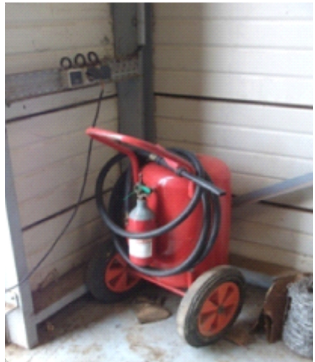
Figure 31 New Fire extinguishers
