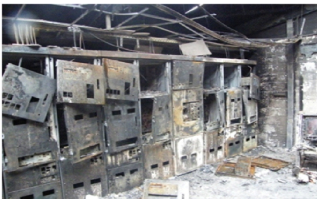
Damaged control equipment & switch gear at Kotu Power Station (source: PURA) 2010
