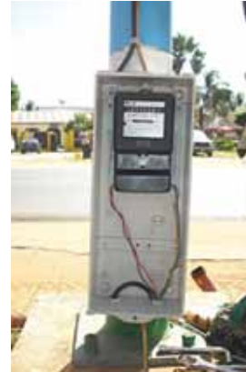
KWH meters wired to each lamp
