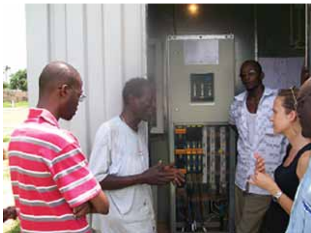
Ownership at Community level, resident of Batokunku explaining the Turbine to a group of visitors
