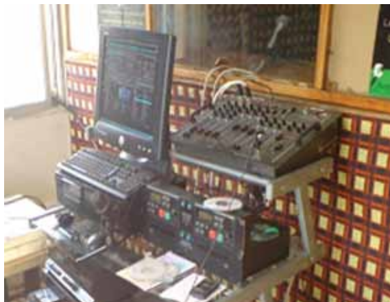
Control room and Studio
