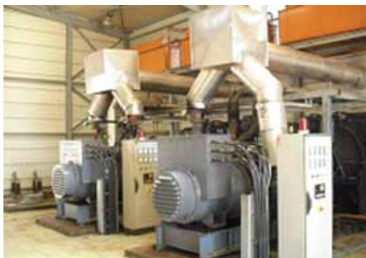
2MWA Power Station in Basse
